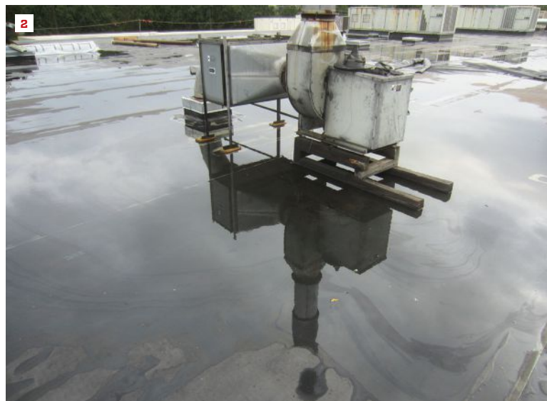
Roof deflection caused by the weight of mechanical equipment that wasn't accounted for in the original design can lead to ponding.
