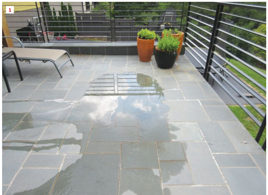
As shown on this exterior deck over habitable space, inadequate drainage caused by the deflection of a low-slope roof can lead to ponding.
