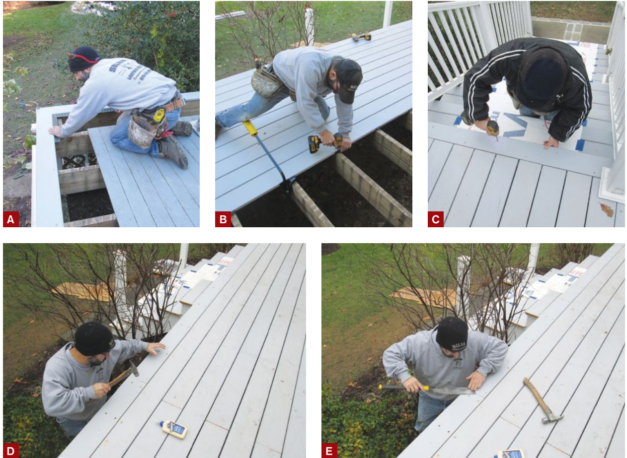
Figure 3. Working from the old decking, the author installed the picture-frame border using \frac{5}{4} \times 6 square-edged decking (A). The field decking was grooved for hidden fasteners (B). After face-screwing the border and treads to the framing (C), the author filled the countersunk holes with plugs cut from the same material (D). Then he flush-cut the plugs (E), sanded them smooth, and used a touch-up paint to color-match the plugs to the rest of the decking.
