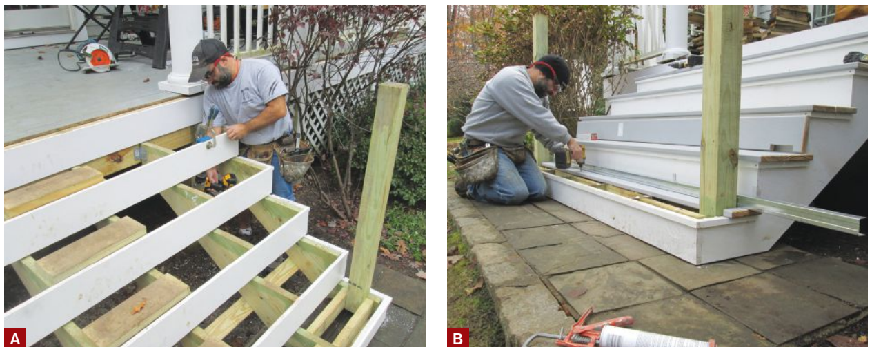
Figure 2. The author reframed the front stairs, cutting new stringers and installing a new dropped header to help support them (A). New \frac{5}{4} \times 6 deck boards were face-screwed to the framing after the PVC skirts and risers were installed (B).
