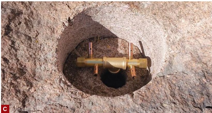
Figure 3. Along with the burners installed in the two boulders, there are also two ground-level burners (A). The black steel gas supply lines run through 2-inch-diameter holes drilled through the boulders (B). Rated at 50,000 Btu each, the assembled brass burners will be covered by porous lava rock (C).
