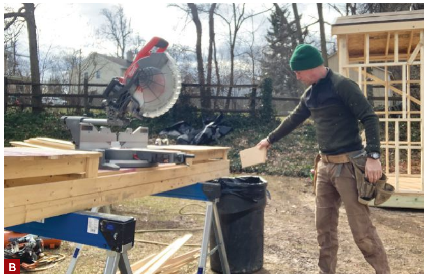
Figure 1. The ability to roll a stack of lumber around instead of moving it board by board contributes to efficiency (A). Placing a trash can to collect offcuts saves the time and energy needed to pick them up off the ground (B).
