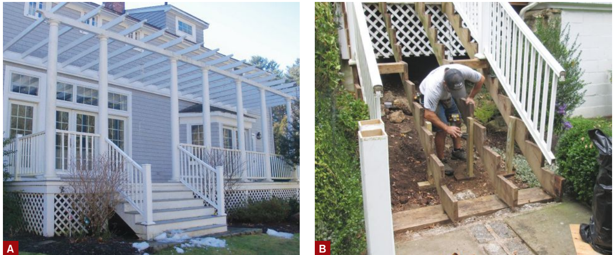
Figure 1. While the original porch framing was sound, the worn and weathered decking needed replacement (A). Part of the repair strategy was to retain the stringers for one set of stairs but pour a new landing pad to support them (B).
