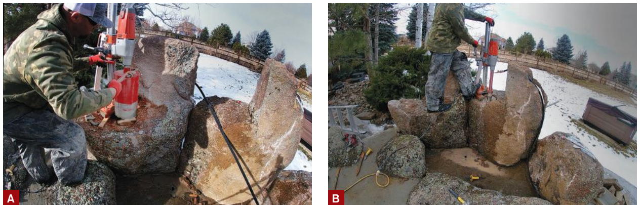
Figure 2. The author carved 8-inch-deep recesses into the tops of the boulders with a 10-inch-diameter core bit to house the burner assemblies (A). Then he drilled 2-inch-diameter holes down through the recess to connect to holes drilled horizontally through the backs of the boulders for the gas lines (B).
