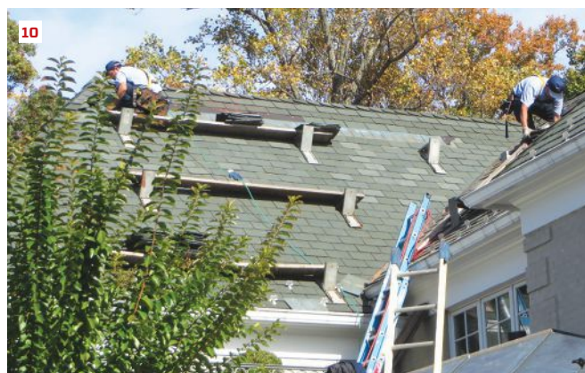
On another project, the author's roofer was not careful with mixing the bundles, and the roof looked odd after 10 years (9). Per the client's request, the shingles were carefully removed, mixed, and reinstalled over new underlayment (10).
