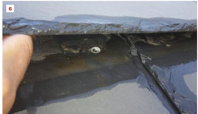
Installing slate without the correct overlap can allow water to wick under the shingles and corrode fasteners, particularly on low-pitched roofs (6). Also, long-lasting fasteners should be used; electro-galvanized nails corrode quickly if they stay wet.
