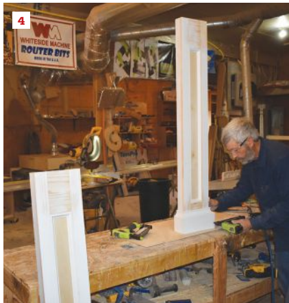
The author used pocket screws to fabricate the frames for the pilasters (2), then built them out to a 2-inch depth with 1¼-inch-wide rippings inset slightly from the frame edge, which he later flush-trimmed (3). After fastening the panels to the frame and adding the panel mold, he installed base mold, which he ripped to a 5-inch width (4).
