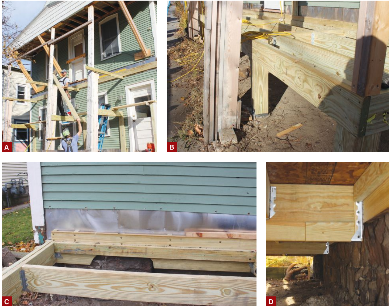
Figure 1. The author shored up the porch roof, then hired a demo company to remove the existing two-story porch (A). The new porch was conventionally framed with pressure-treated lumber, with the joists parallel to the front of the house (B). The oversized ledger was blocked out away from the wall (C) to clear the house's irregular stone foundation (D).
