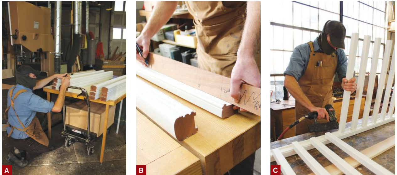
Figure 4. The author shaped and painted the railing parts in his shop (A), then used a story pole to lay out the baluster locations (B). He started assembly by pinning the balusters to the dado cut in the underside of the middle rail (C).
