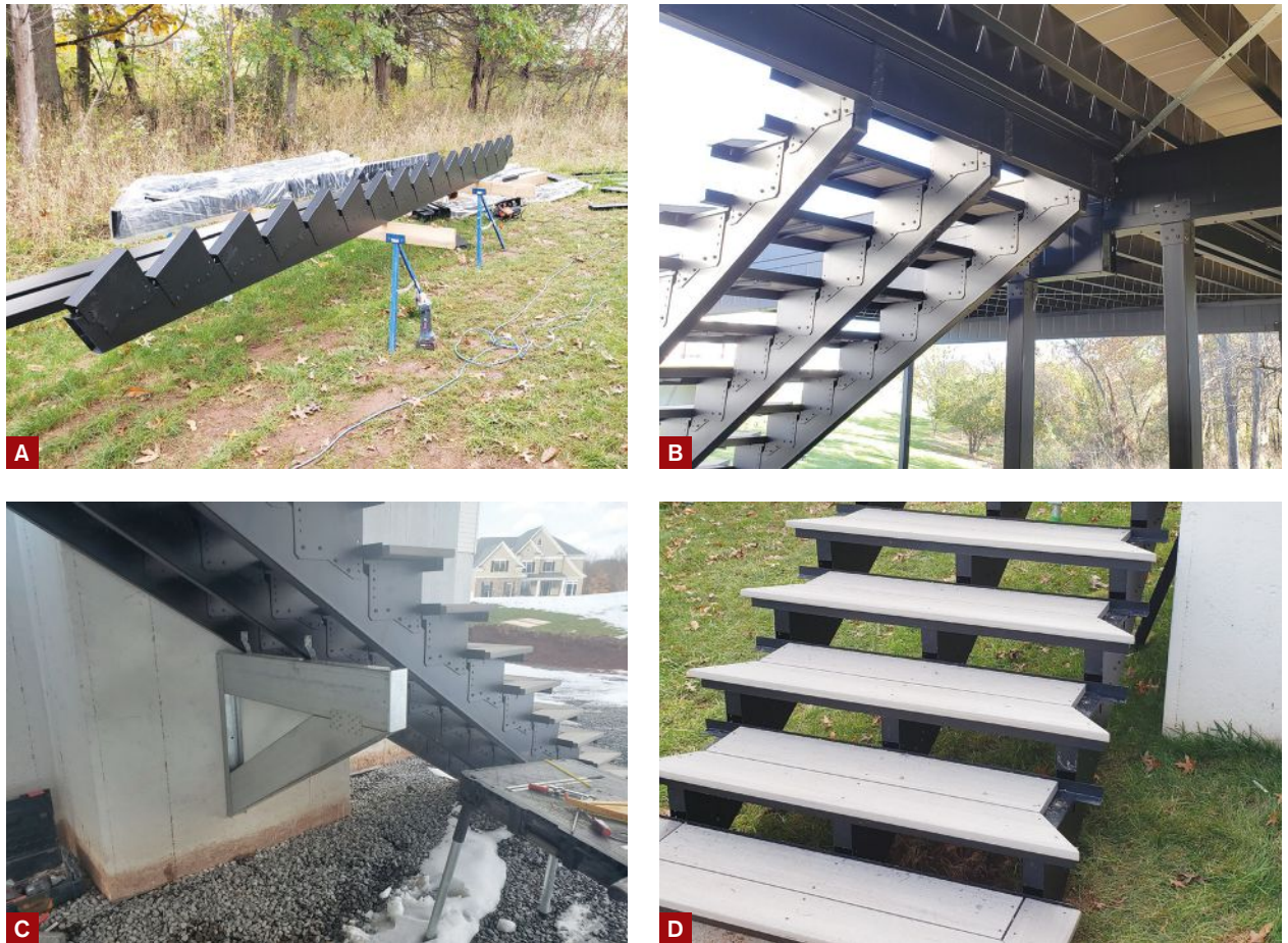
Figure 6. To build stair stringers, proprietary brackets are fastened to standard joists (A), which are then fastened to the framing with adjustable strap-like hanger brackets (B). A midspan bracket enabled the author to build the stairs before the hardscaping was completed (C). Wider, 7-inch deck boards created an overhang for the two-board treads (D).
