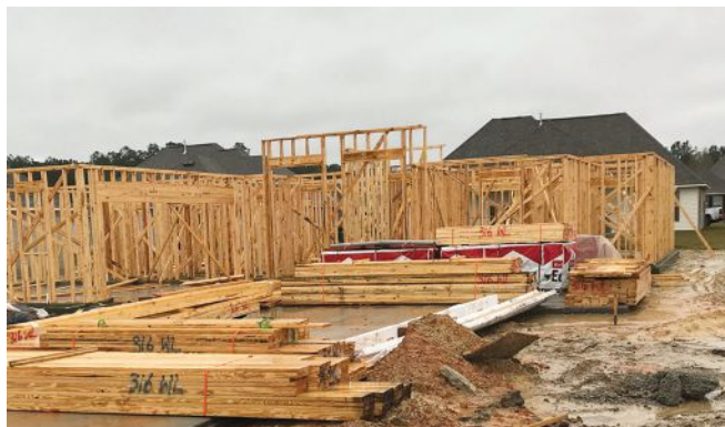
Wet framing and a short building cycle is a good recipe for nail pops, drywall cracks, and other callbacks.
