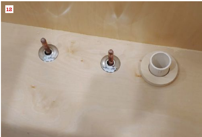
A jig speeds installation of cabinet hardware (10). When a cabinet that has already been drilled for plumbing lines has to be shifted slightly, a wood trim ring can be fabricated to cover the enlarged hole around a drain line (11, 12).
