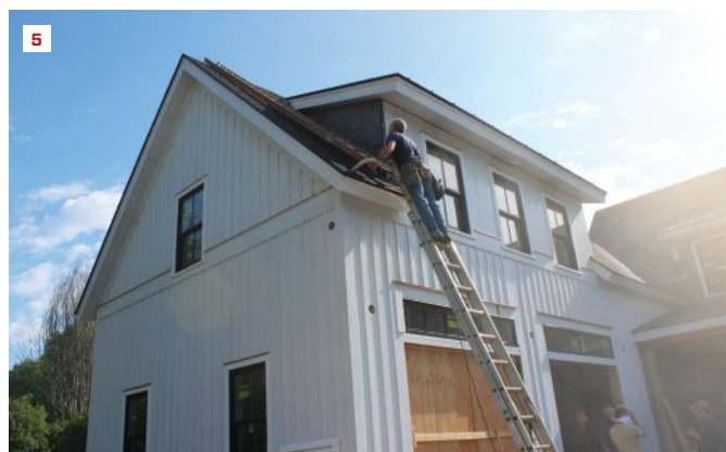
Co-author Jim Bradley points to smoke leaking from double-hung windows in living space above the garage (4). After checking the window openings and dormer framing, workers determined that the window units themselves were leaking (5).
