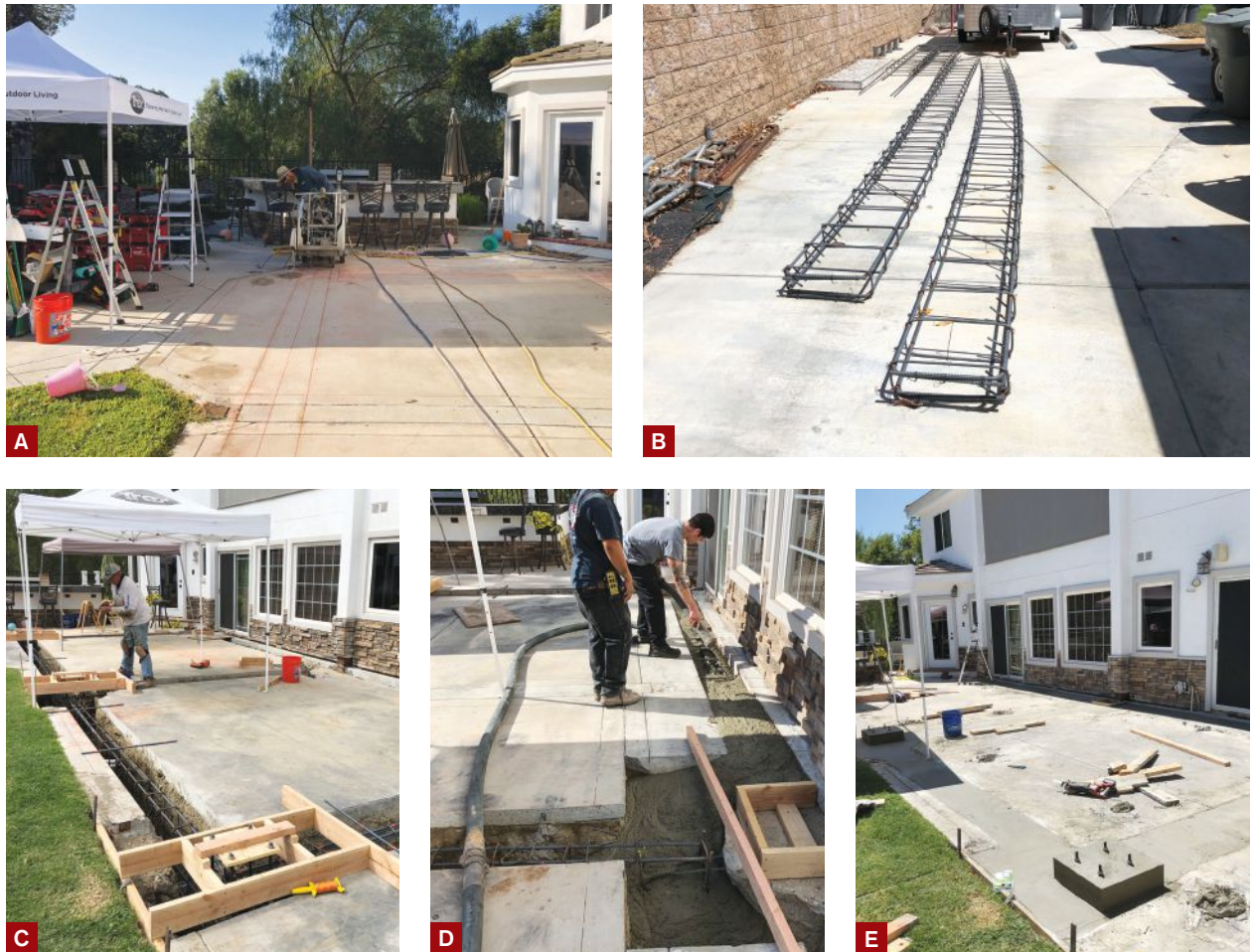
Figure 1. A 12-inch-wide slot was cut through the concrete patio for the new grade-beam footing engineered to provide lateral support for the freestanding deck (A). The rebar cages were partially assembled, then delivered to the site (B), where the crew finished tying them together after the steel reinforcement was placed in the 24-inch-deep trenches. The crew carefully formed up the piers for the deck's steel support columns to ensure that the deck ended up at the proper elevation (C). Rebar dowels were added to the cut edges of the patio to tie the concrete slab to the grade beam after the new concrete was poured (D). Before the steel columns were installed, nuts were threaded onto each of the pier's four anchor bolts, which would later be used to fine-tune the height of the columns and adjust them for plumb (E).
