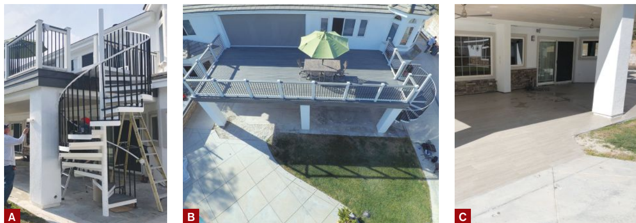
Figure 8. The new stucco finish on the columns and soffit was painted to match the existing house (A, B). To wrap up the project, the old concrete patio was prepped to receive new plank-style patio tiles patterned to match the deck's wood ceiling (C). Though not shown in the photos, a new door that provides access to the upper level was installed in a follow-up project.
