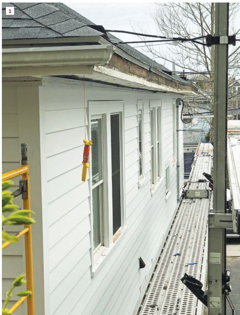
Roller coaster eaves. This house got an entirely new face lift, which included a tear-off and replacement of all the old siding and trim. But rather than demolish the eaves and rebuild them, the author chose to lay over the old eaves with a new assembly.
