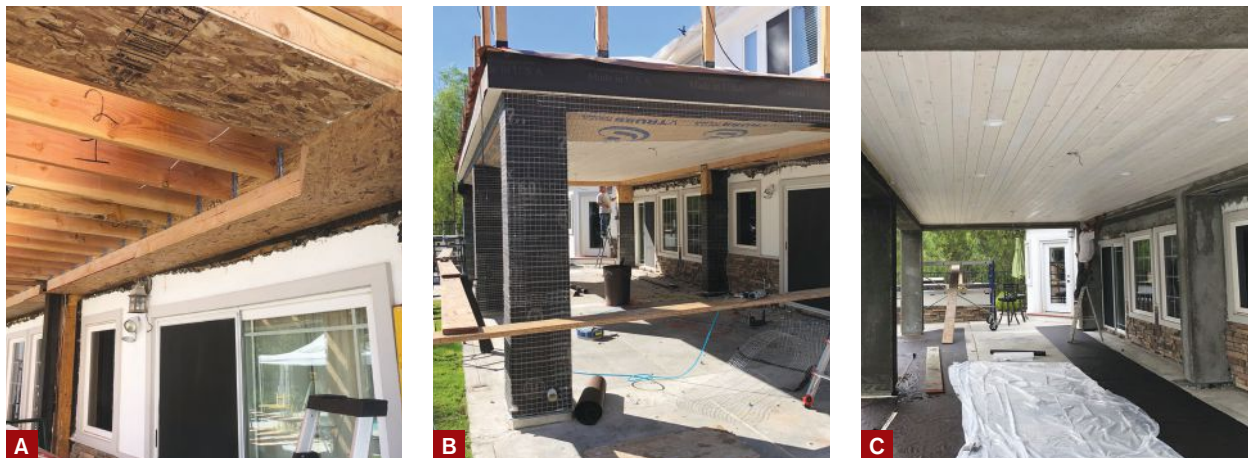
Figure 5. Underneath the perimeter of the deck, workers framed a soffit and covered it with OSB in preparation for a stucco finish (A). After covering the soffit and boxed columns with building paper and wire lath for the stucco (B), workers installed the tongue-and-groove wood plank ceiling (C). J trim was installed at the corners where the ceiling would meet the stucco to give the installation a clean look.
