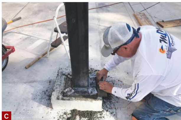
Figure 2. Fabricated by a certified welding shop, each of the engineered steel columns weighed about 250 pounds; a portable contractor's lift was used to hoist them into position on top of the concrete piers (A). The lift would also be used to hoist heavy 7x14 PSL beams into place on top of the columns once the columns had been bolted to the piers (B). Workers turned the nuts supporting the columns with a box wrench to adjust the columns' height and plumb, then packed the voids between the column base plates and piers with non-shrinking grout (C).
