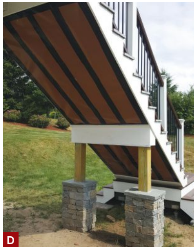
Figure 3. Workers determined the position and elevation of the stair landing with the help of a stringer for the upper flight of stairs (A). The landing was framed with steel and supported by helical piles (B). Steps lead up to the landing from all three sides (C). RainEscape troughs were fastened to the stair stringers so the underside of the stair could be finished with beadboard (D).
