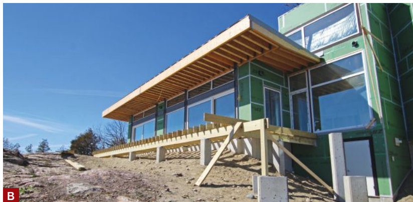
Figure 1. The bedroom-office wing was "floated" on the piers. Here, the deck was being framed on the home's elevated southeast corner (A). The larger deck off the main living area was close to grade and supported by shorter piers (B).
