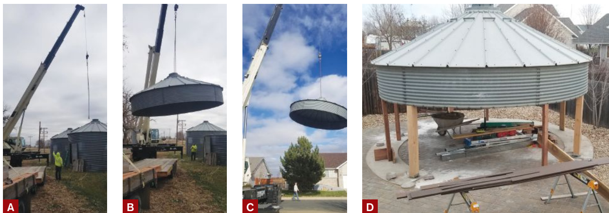
Figure 2. After most of the bolts holding the grain silo sections together were removed, a crane lifted the roof and upper section from the rest of the structure (A) and set it onto a flatbed trailer (B). At the client's home, the silo roof was hoisted over the house (C) and set gently onto temporary 4x4 posts. Later, permanent 6x6 posts were installed (D).
