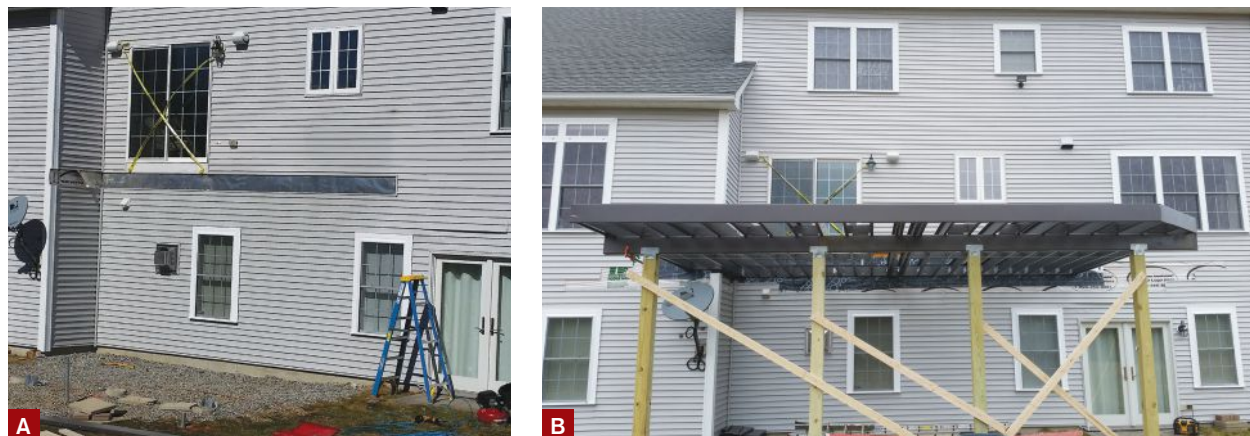
Figure 1. In the first phase of the project, workers removed the existing deck and installed new helical piles (A). The new deck was framed with Trex Elevations light-gauge steel, supported by 6x6 PT posts that bear on the helical piles (B). On the right-hand outside corner of the deck, the framing has been clipped at a 45-degree angle to accommodate the stairs leading to the upper level.
