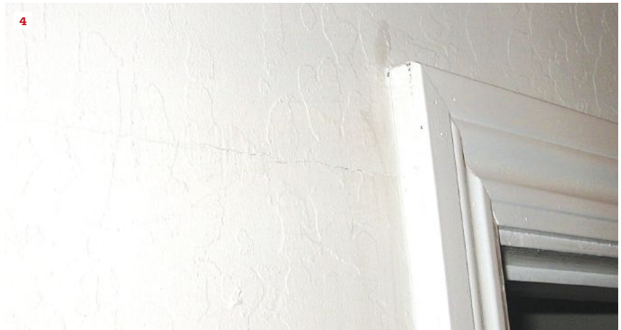
Panel joints placed too near window and door corners will tend to crack as the lumber in the header and other framing around the openings shrinks.
