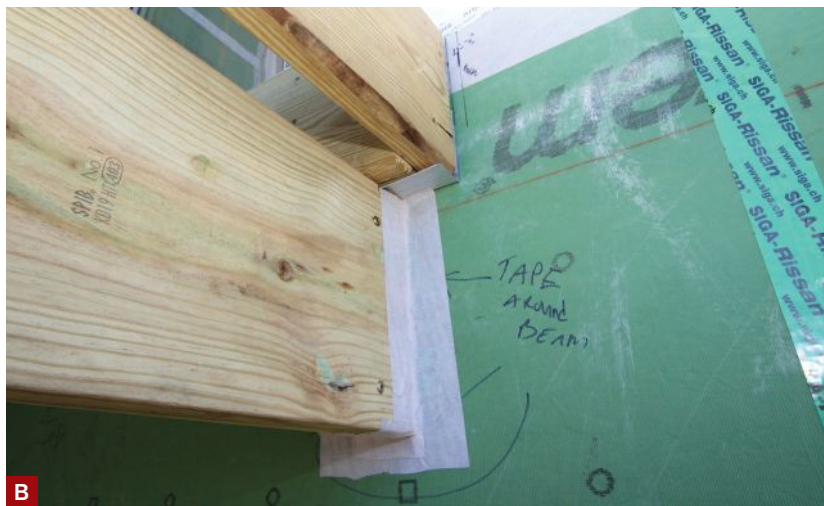
Figure 2. Ledgers were lag-bolted through spacers to the elevated floor's triple LVL rim beams spanning the piers (A). Fentrim flashing tape was used for both water- and air-sealing. Here, it air-seals a deck beam pocketed into a wall (B).
