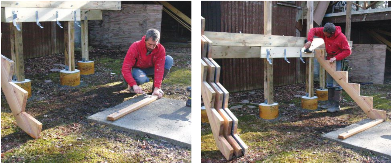
Figure 1. After pouring the concrete for the strip footing and stair landing, the author uses anchor bolts to connect a 2-by PT cleat to the footing (above left). When installing the end stringers, he fastens them to the cleat with structural screws (above right). The middle stringers will be notched to fit over the cleat.
