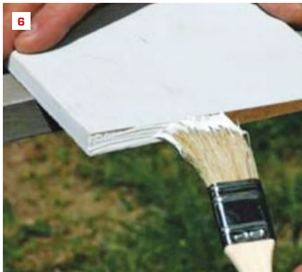
Unprimed siding won't hold paint for long. This paint job on a new addition (4) is less than five years old. Factory-installed primer is better than no primer, but it won't block the bleed-through of extractive oils in cedar (5). An additional coat of acrylic primer is needed before the finish coat. All field cuts need to be primed before installation of all siding and trim (6).
