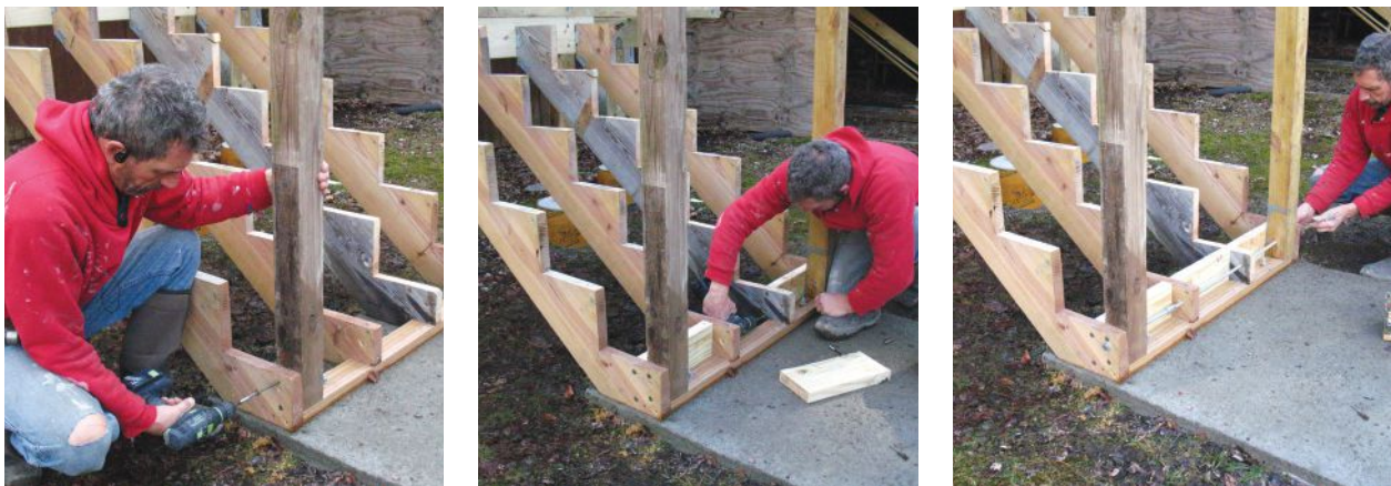
Figure 2. The author screws the guard posts to the stringers (above left), then installs a row of blocking that fits tightly between the stringers (above center). A 1/2-inch-diameter galvanized threaded rod that fits through prebored holes in the posts and stringers ties the assembly together (above right).
