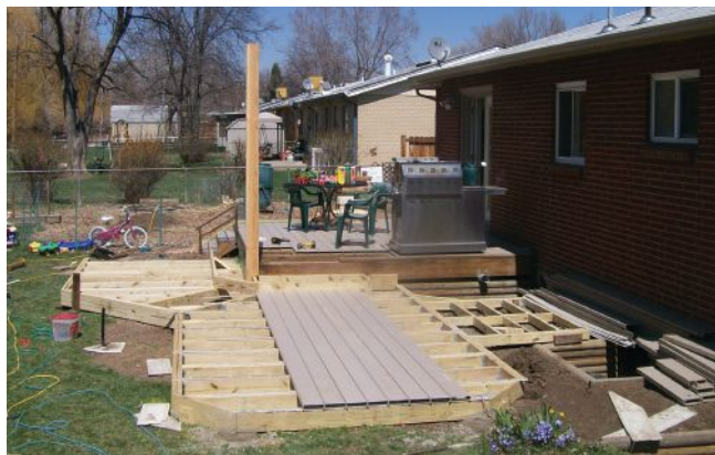
A grade-level deck doesn't need to be supported by a concrete foundation, as long as the deck is not connected to the house framing.
