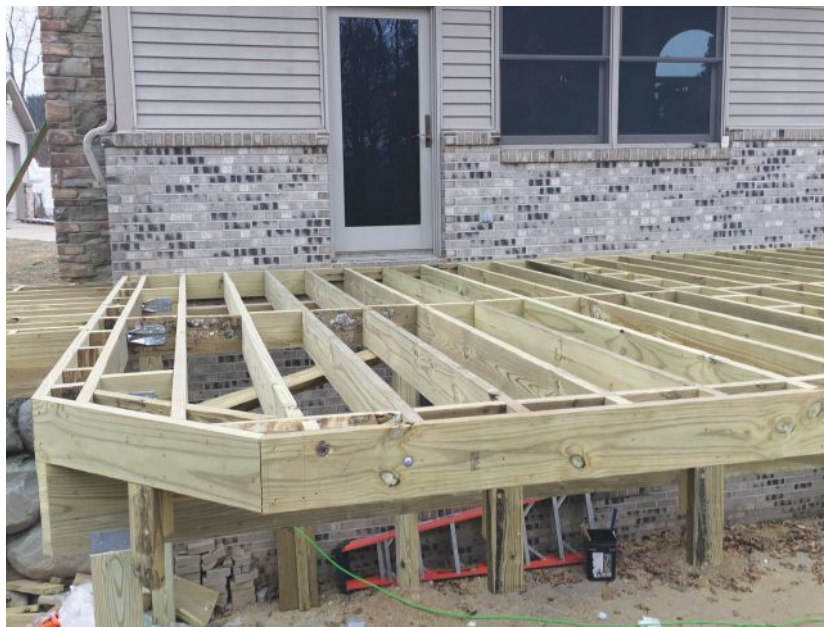
Figure 1. Vertically oriented for drainage, blocking has been added to the deck framing in preparation for installing a picture-framed border.
