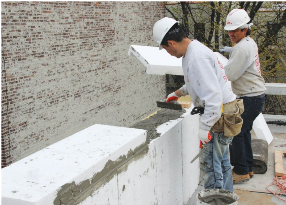
Parapet walls for low-slope roofs can be insulated with a rigid-foam wrap that integrates into the wall insulation and the roof insulation of the building, as shown here in a Passive House project from 2016.
