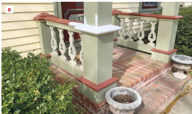
With two coats of paint and an annual inspection, this repair should last indefinitely (9).
