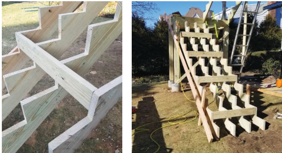
Figure 4. To make the stringers straighter and stronger, the author notched the middle stringers and installed 2x6 blocking (far left). Located every few steps, the stringer blocking keeps the tops of the treads aligned and ties the assembly together into a solid unit (left).
