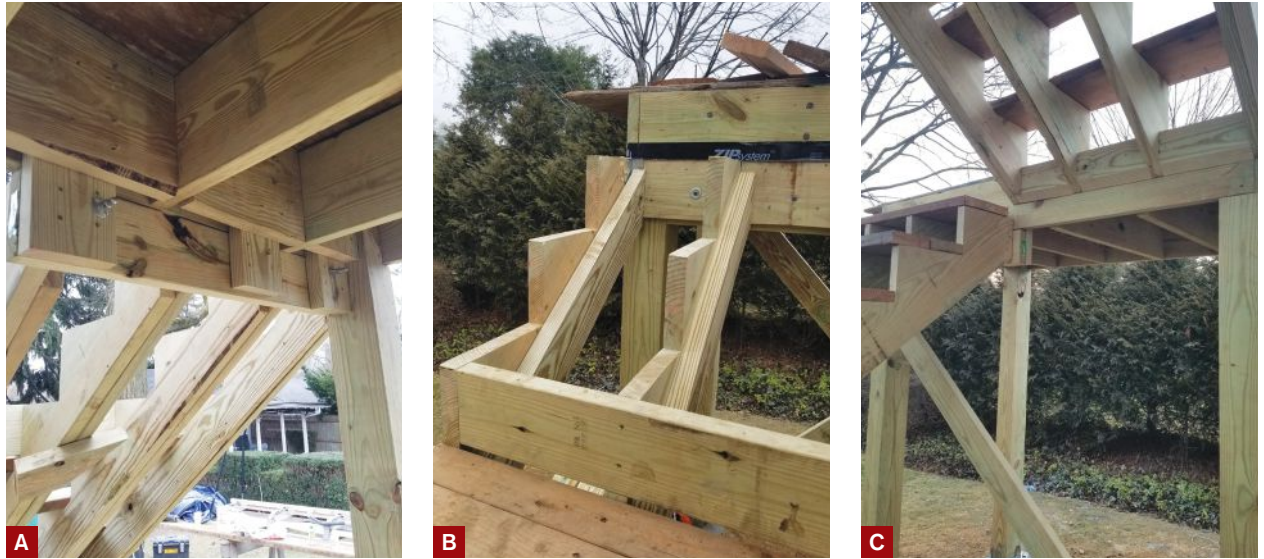
Figure 3. The stair stringers were hung from a 2x6 connected to the rim joist with vertical blocking and a combination of structural screws and ThruLok bolts (A). The author reinforced the stringers with sistered 2x6s (B) and reinforced the connection between the upper stringers and the landing platform with blocking (C).
