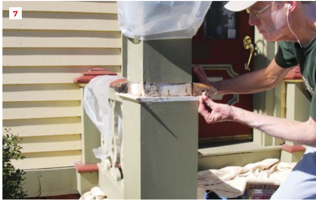
Before the miters are assembled, the author drills a hole and inserts a Bor8Rod that will provide an extra measure of insurance against rot (7).
