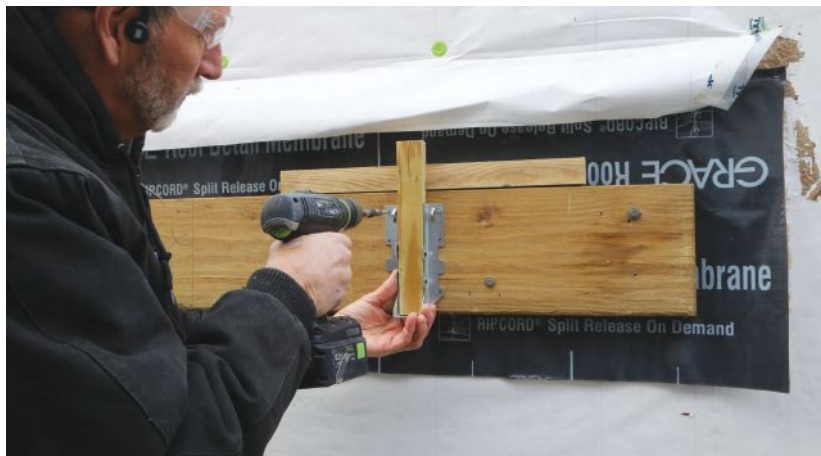
Figure 5. The author prefers to install joist hangers prior to hanging joists, using a site-built T-jig to quickly and accurately place the hangers. When using this method, be sure that the joists are uniformly sized.
