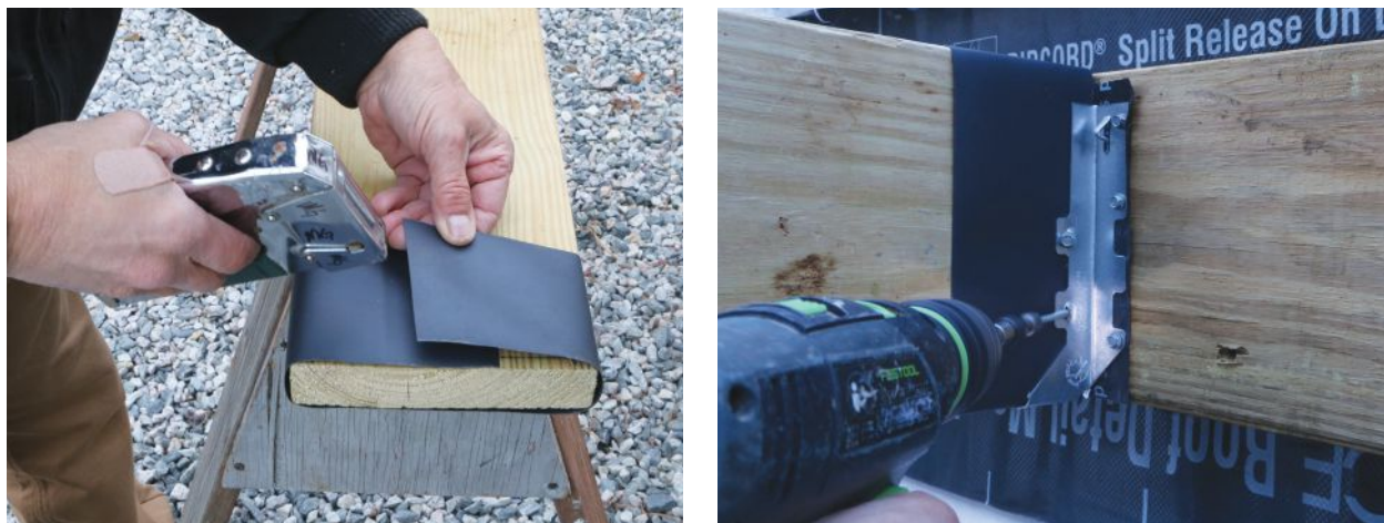
Figure 3. Applying a staple-on isolation membrane or a self-adhering membrane to joist ends (above left) and the ledger (above right) reduces the rate of galvanic reaction between the treated lumber and the metal hanger.
