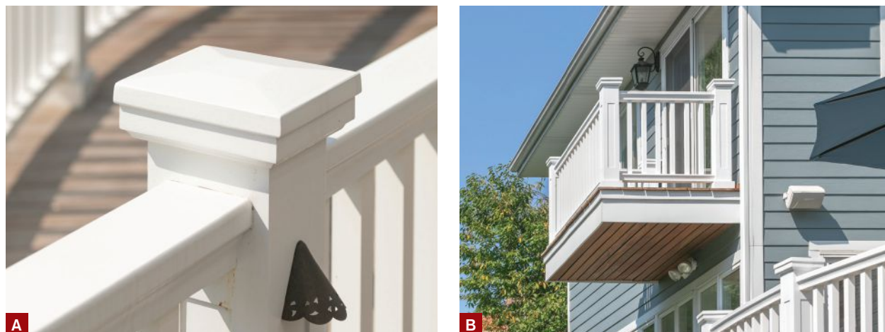
Figure 4. The author sanded the sleeves, caps, and bases and gave them a coat of 100% acrylic latex paint, then assembled all of the components on the jobsite (A). The rails were fastened to the posts with 4-inch-long screws (B).
