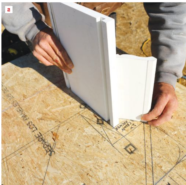
Visualizing the details of eaves is easier with a full-scale drawing. For this complex eaves with crown molding, the builder uses a section of the molding along with a piece of 1-by stock to ensure a proper layout (2).
