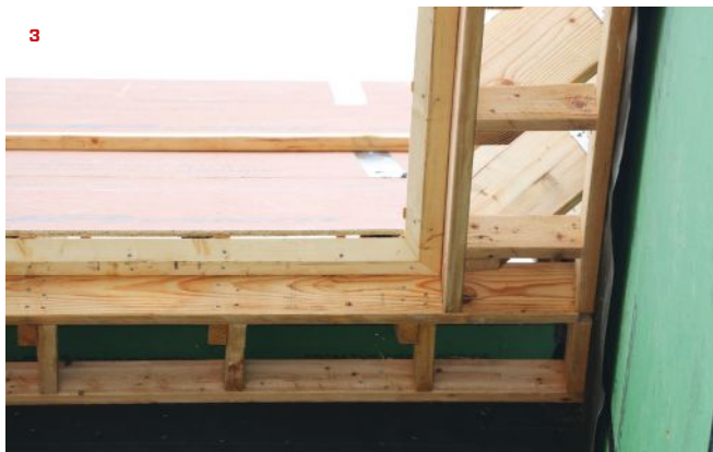
Seen from below, blocking between the subfascia and the wall adds plenty of nailing surface for attaching a wider soffit (3).
