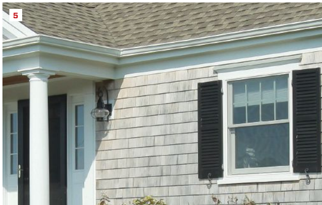
A frieze board (5) captures the top edge of the siding while closing the joint between the soffit and the wall.
