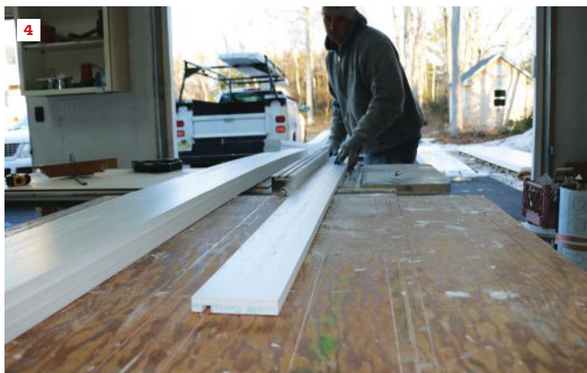
To join the fascia to the soffit, this crew member runs the 1-by fascia material through a table saw to create a dado groove (4).
