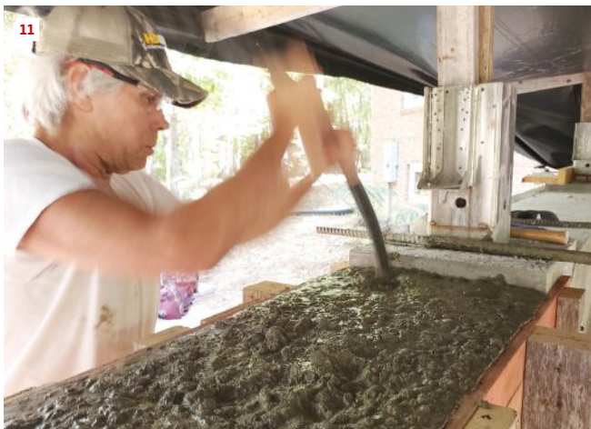
Choose concrete with a 4-inch slump for flatwork (9). Use a stiffer mix of 2 to 3 inches for deeper work such as this footing (10), then consolidate the mix with a vibrator (11).
