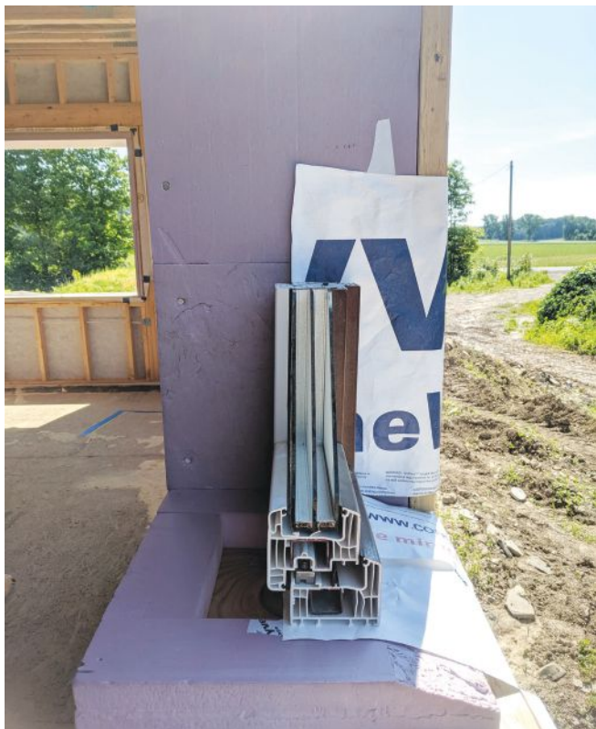
A mockup of the author’s window installation shows the insulated window buck and the window’s location near the wall’s center of mass.
