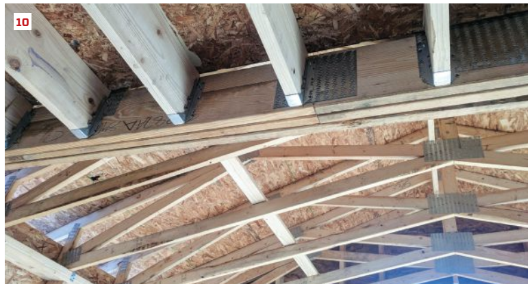
A scissors-truss roof abuts a carrying beam for a floor system (8), as does this flat ceiling truss (9). The leakage pathway is visible when the framing junction is viewed from the other side (10).
