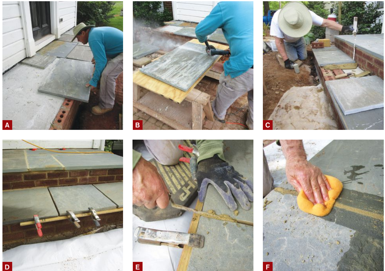
Figure 2. The author dry-fit the bluestone pavers (A), numbering them to keep track of their location, then trimmed them to size as needed with a diamond blade mounted in an angle grinder (B). The pavers were set in a thick bed of type S mortar (C). After the mortar bed cured, he grouted the 1/2-inch-wide joints with the same type S mortar. A strip of wood clamped to the pavers where they overhung the brickwork supported the grout while it cured (D). The author used a tuck pointer to pack the joints (E), and he cleaned up the joints afterward with a damp sponge (F).
