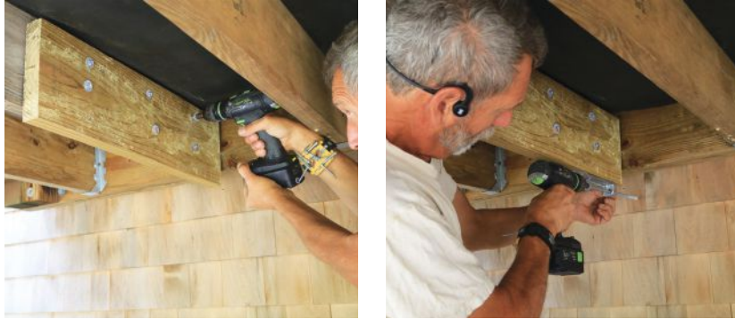
Figure 10. Blocking can be installed to help align the hardware with the deck and house framing. Here, the author fastened the block to the joist with SST TimberHex HDG screws (above left) before installing the DTT1 tie (above right).
