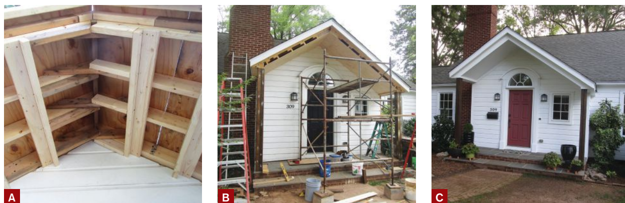
Figure 6. The author fastened collar ties to the rafters and ridge with structural screws (A) and blocked out the roof framing with 2x4s to provide nailing for the plywood ceiling (B). The completed portico was painted to match the house (C).
