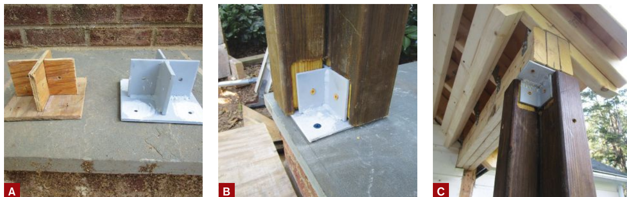
Figure 5. A local supplier fabricated the custom steel column brackets based on a plywood prototype supplied by the author (A). Each column consists of four 3x3 posts connected via the brackets to the masonry stoop (B) and beams (C).
