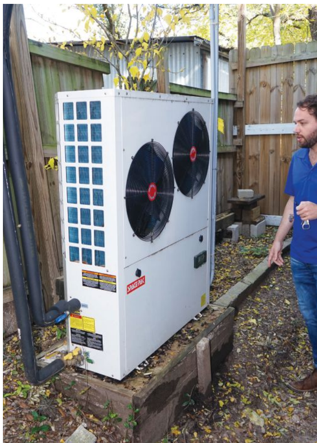
Outside the building, a 3-ton SpacePak Solstice air-to-water heat pump dumps excess heat from the building to the outdoor air—just one of many possible solutions that are possible with radiant cooling.
