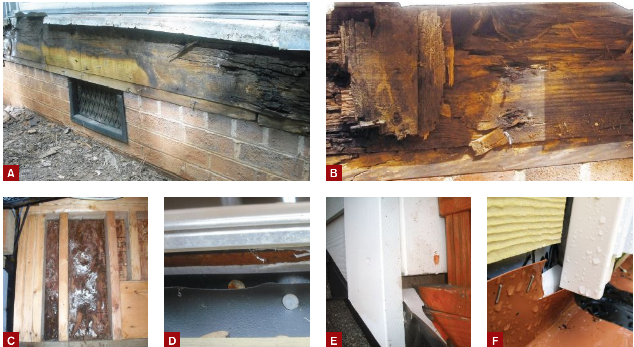
Figure 5. The sheathing and band joists on these homes (A, B) are in rough shape, thanks to moisture intrusion from their decks, and require replacement. Improperly installed ledger flashing on a one-year-old deck was the cause of this water damage (C). Flashing is often improperly installed underneath door thresholds (D) and where ledgers intersect with other building components, such as a roof (E). During a new-home inspection, the author discovered flashing that hadn't been integrated with the water-resistant barrier underneath the home's siding (F).
