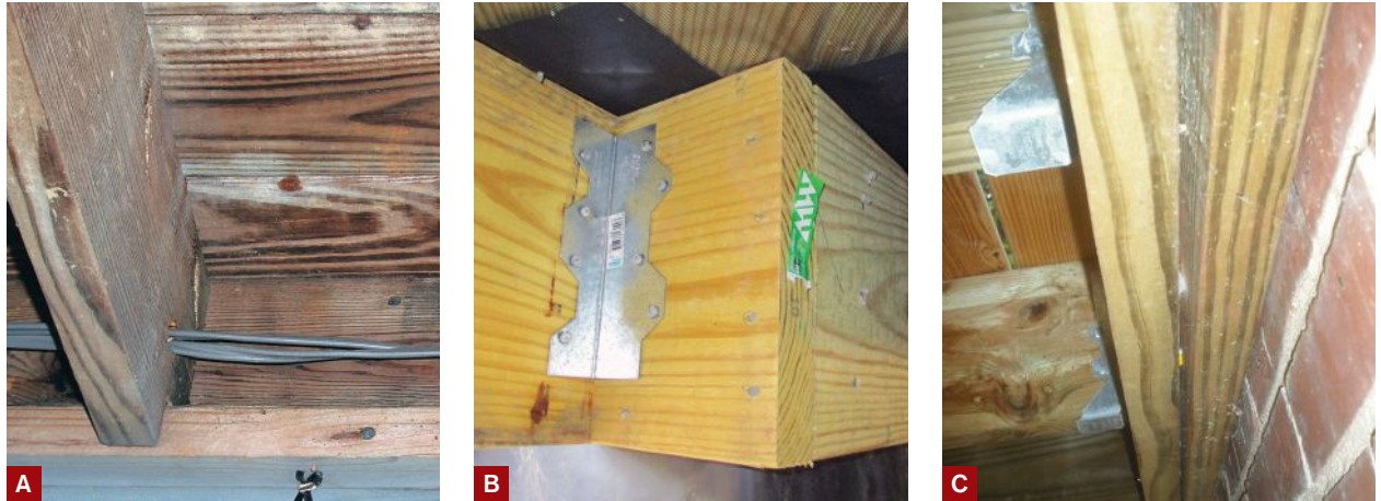
Figure 1. Older decks frequently have ledgers that have been nailed rather than screwed or bolted to the house (A), but the author sometimes finds this problem on recently built decks too (B). Note the nailed double-ledger connection, which is in the process of separating, in photo (C).
