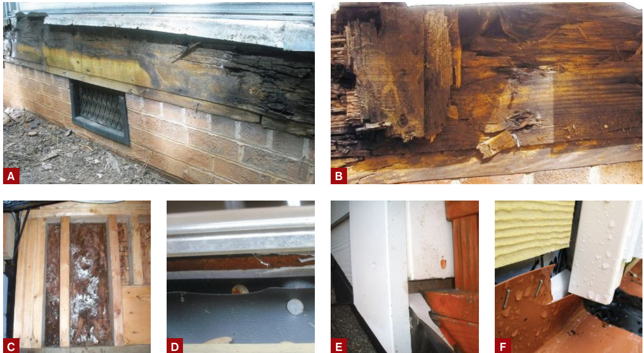
Figure 5. The sheathing and band joists on these homes (A, B) are in rough shape, thanks to moisture intrusion from their decks, and require replacement. Improperly installed ledger flashing on a one-year-old deck was the cause of this water damage (C). Flashing is often improperly installed underneath door thresholds (D) and where ledgers intersect with other building components, such as a roof (E). During a new-home inspection, the author discovered flashing that hadn't been integrated with the water-resistive barrier underneath the home's siding (F).
