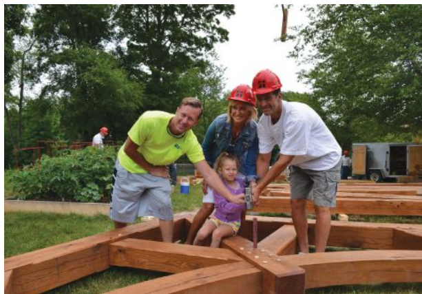
Family and friends are always invited to help assemble the company's timber frames. Here, the pavilion's purpleheart "giving peg" is being hammered into place.
