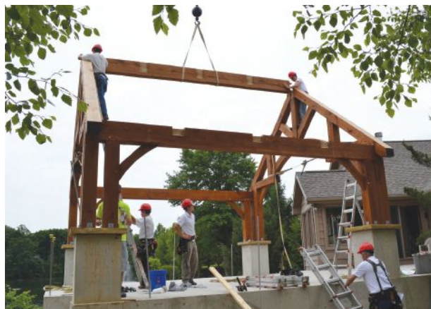
A 6x12 ridge beam ties the two end trusses together. For temporary protection, the pieces were coated with a water-based finish back at the woodshop.
