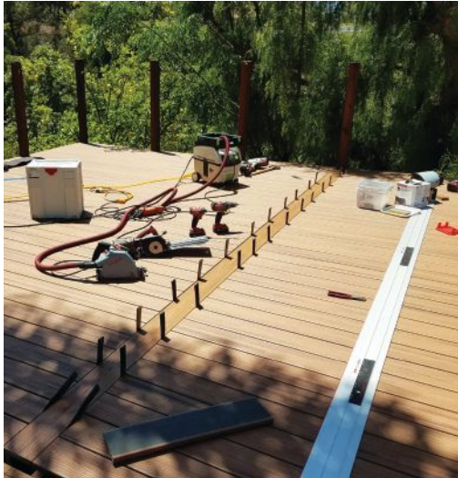
Figure 2. You can avoid the need for butt joints by installing a seam board in the middle of a wide deck. Here, California deck builder Michael Walter used shims to create consistent gaps between the seam board and the ends of the deck boards.
