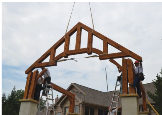
Crafted from 8x8 white-oak timbers with 8x12 plates, the 18-foot-wide frame has a 10-in-12 pitch roof. Above, a king post-and-strut truss is being lifted into position.
