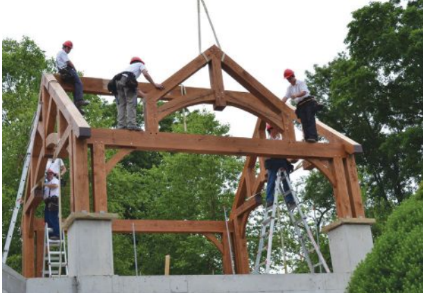
After OakBridge workers installed the dormer face truss and remaining 8x8 rafters to finish up the frame, a local crew installed a white-pine tongue-and-groove roof deck.
