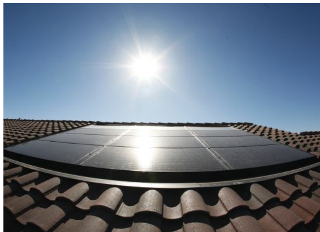
Solar panels on the tile roof of a Meritage home
