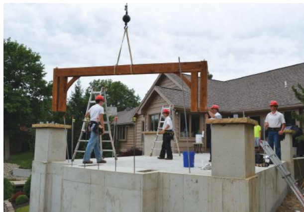
Once the components have been assembled on the ground, a crane lifts them into place, where they are installed by the OakBridge team.
