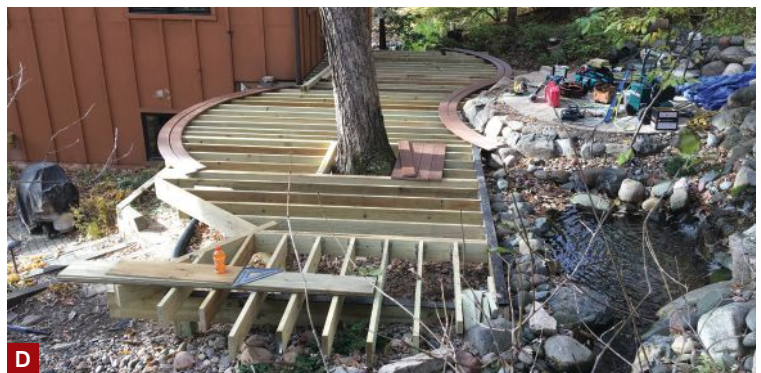
Figure 1. The author installed cantilevered joists over dropped beams, running the joists long (A) and then laying his heat-formed borders over the joists (B) to define the curves. After the joists were marked and cut to length, workers installed blocking as needed (C) and framed the opening around the tree trunk (D).
