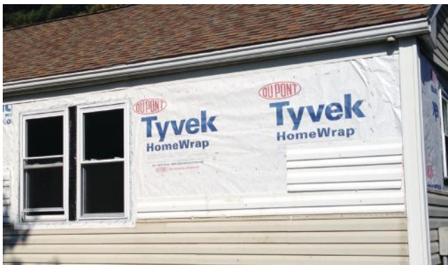
The author installed a working drainage plane using tape-sealed housewrap to keep the house walls dry, flashing below the fascia trim and pulling the roof drip edge away from the roof to direct rainwater into the gutters.
