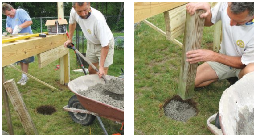
Figure 3. In a top-down framing approach, the deck is framed on temporary supports (above left), which allows for more accurate placement of the footings (above right). In some jurisdictions, the approach allows for a single inspection visit for framing and footings.
