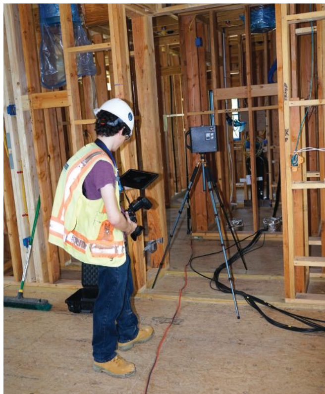
A Multivista technician uses a Matterport scanner and an iPad to create an accurate, photo-realistic virtual model of a Risinger Homes building under construction in 2018. At the same time, the tech is taking high-resolution still photos of some locations, which can be keyed to the virtual model of the building.
