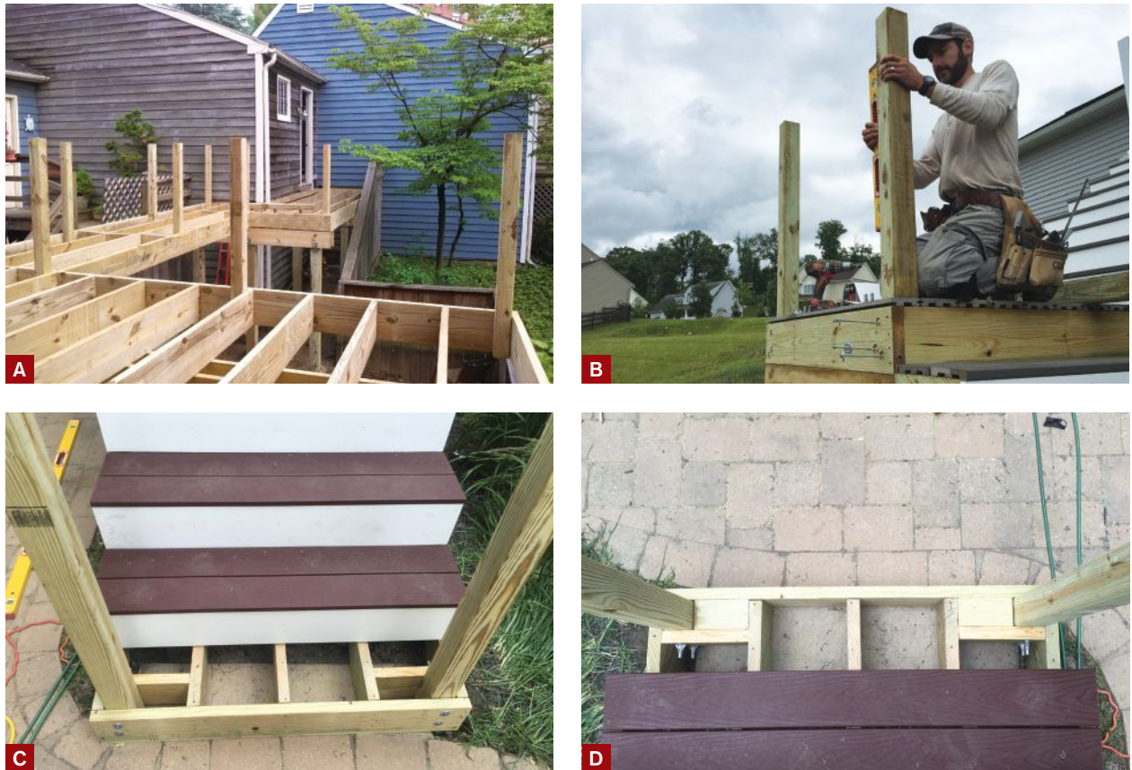
Figure 5. Tacking guard posts in place as the deck is framed (A), then going back later to install blocking and plumb the posts all at once (B) can help speed installation. Both vertical (C) and horizontal (D) blocking can be used to reinforce the connection between stair guard posts and the stair stringers, though remember that blocking installed on the flat should be protected from water intrusion with a peel-and-stick flashing membrane.
