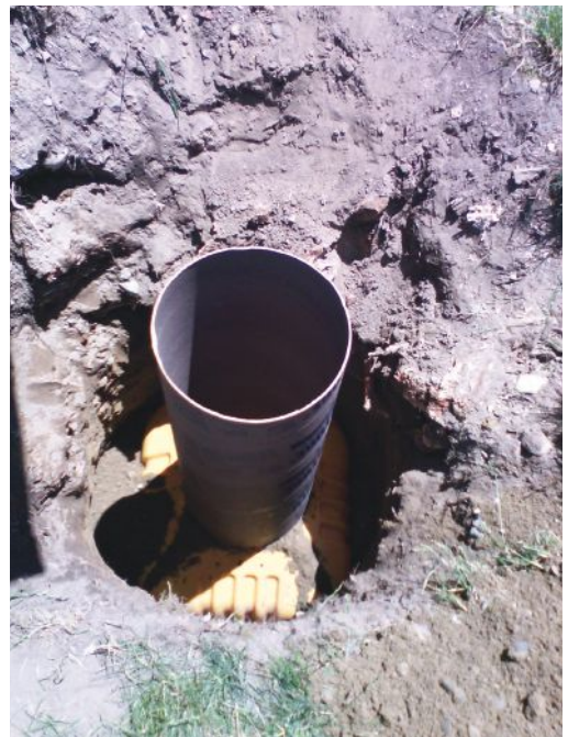
Figure 1. Some building inspectors may allow you to skip certain jobsite inspections as long as you can provide them with clear photos showing that your work meets local code requirements, such as footing depth (top). Not having to wait for the inspector will keep the job moving. Another benefit to taking photos is that you will have documentation of the details used in the construction of the deck (right).
