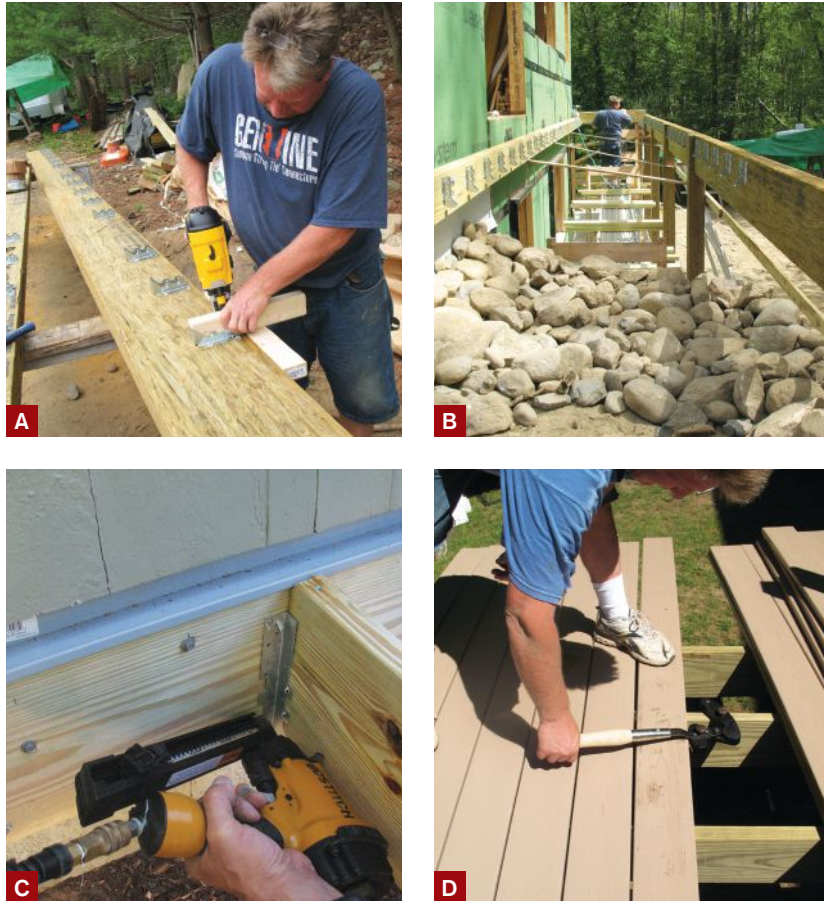
Figure 2. Joist hangers can be preinstalled on the framing, using a simple joist-hanging jig to accurately position the metal hardware (A). After the rim joist and ledger have been installed, joists can be quickly dropped into place (B). Key specialty tools include metal-connector nailers (C) and board benders (D).
