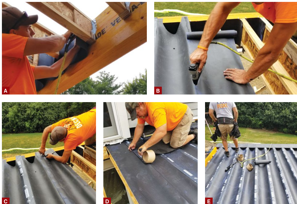
Figure 2. The waterproofing process begins with cutting 14-inch-by-18-inch bibs from 40-mil EPDM rubber waterproofing membrane, and stapling the bibs to the front of the beam (A). A worker then staples tapered EPDM troughs to the joists, bedding the troughs where they overlap on top of the joists into a thick bead of neoprene sealant (B). After cutting away excess material to allow water to flow freely down into a gutter installed underneath the rim joist (C), a worker covers the tops of the joists with SAF flashing tape (D). Around the perimeter of the deck, another membrane layer is installed over the top of the LVL framing to direct water back into the troughs (E).
