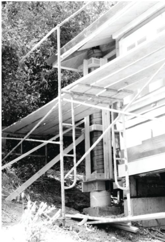
The stepped concrete column (whose formwork is visible behind the scaffolding) was costly to construct for several reasons, including complexity and difficult access. Most impactful, the column was to serve as a prominent finish item, so all forming and concrete installation had to be meticulously controlled.
