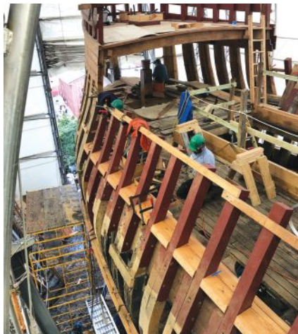
Clockwise from top left: Mystic Seaport shipwrights Brett Land drilling holes for trunnels, Anthony Daniels fairing the hull, Greg See installing waterways, and Anthony Matt hand-planing a plank.
