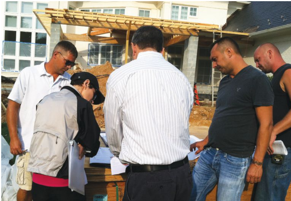
Frequent ad-hoc meetings between project managers, production managers, and trade contractors to iron out critical details help to keep jobs moving and on schedule. Here, metal roof details are being discussed with the roofing contractor.
