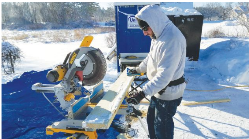
The author supplies his workers with cold-weather gear. When it snows, crews are equipped with snow-removal equipment and pop-up shelters to keep work areas dry and snow-free.
