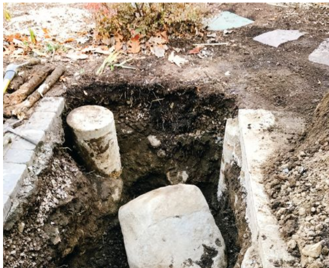
Figure 4. The piers supporting the landing were too shallow, probably due to the boulders that had been buried under the slab (top left). Removing them was a difficult but necessary job (bottom left).
