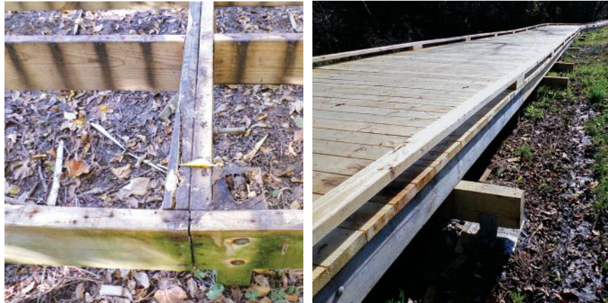
Figure 3. Considerable rot was found in the existing posts supporting the boardwalk (far left). The damaged posts were also replaced with metal anchors, then new 2x6 PT decking was installed to complete the repairs (left).
