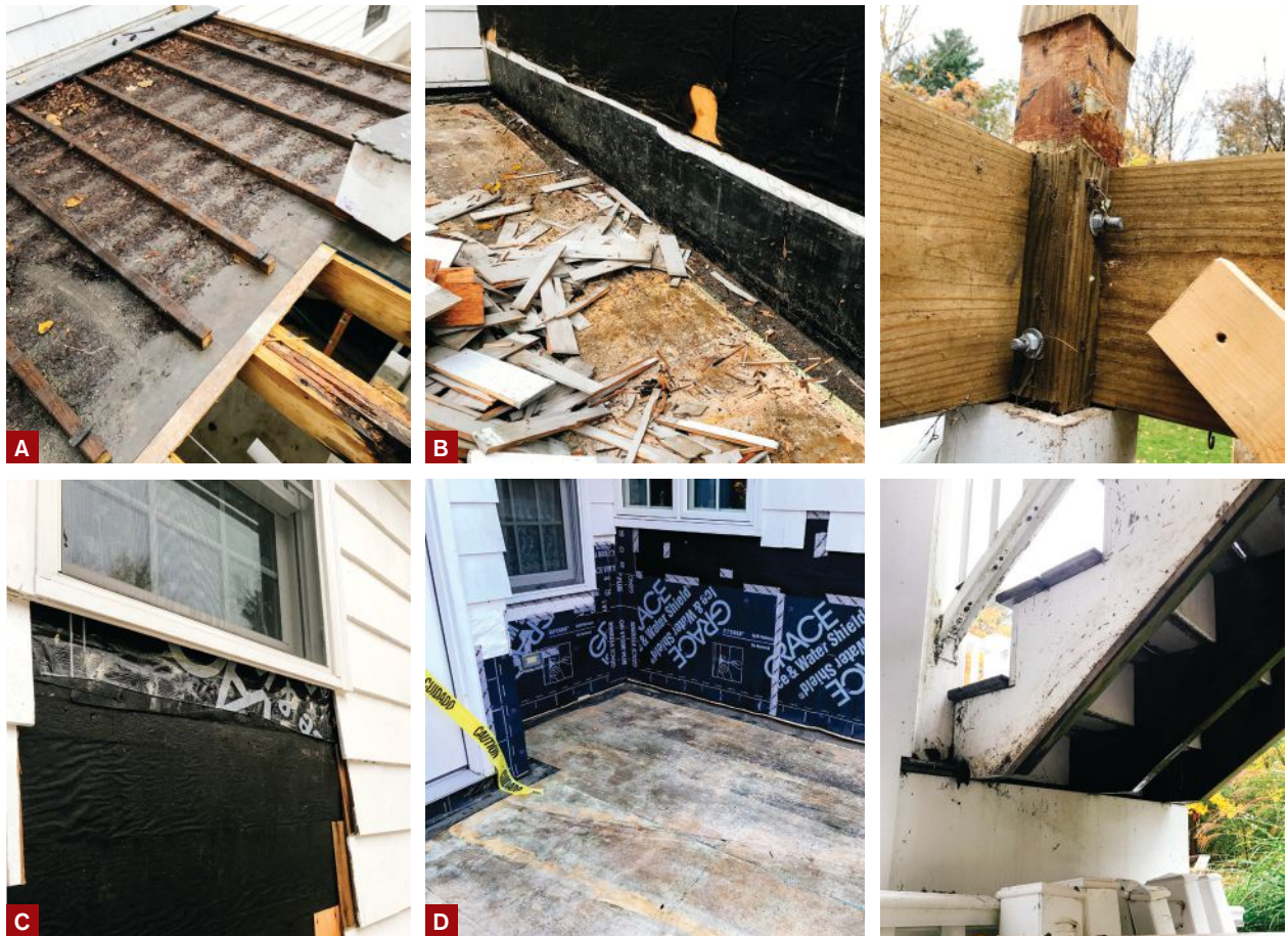
Figure 2. Water that had seeped down into the triple support beam below the posts had caused significant rot (A). The water-resistant barrier (WRB) had been punctured by hundreds of staples, and deck-to-wall flashing was reverse-lapped over the WRB underneath the wall shingles, creating potential pathways for water to penetrate the structure (B). Windows had also been improperly sealed to the WRB underneath their sills, preventing drainage (C). To eliminate these problems, it was necessary to strip the shingles back to the window sills and install a new WRB (D).
