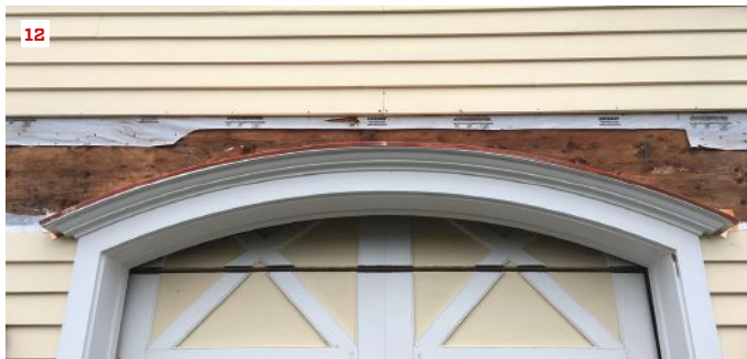
Flashing was shaped with Eastwood shrinker (blue) and stretcher (gray) tools (9). Flashing in the corners helps direct water away from the wall (10). Flashing was installed with minimal nailing; ends were folded down (11). The center seam was soldered (12).
