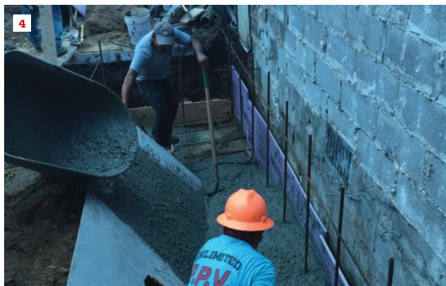
Masons apply brick veneer to the two-story block addition (1). An existing 8x10 bump-out addition was removed prior to construction (2). During demolition, it was discovered that an abutting neighbor’s two-story addition was built on undersized footings (3). New footings had to be poured with concrete wheelbarrowed through the house from a mixer truck parked street-side (4).
