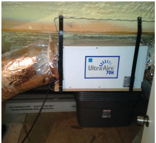
North Carolina builder Tom Dugan installed this Ultra-Aire 70H in his own home. The unit is rated at 70 pints per day and 5 pints per kWh. Dugan tied the dehumidifier into his already installed fan-powered air-mixing duct, which sends air from the home’s highest point down to the ground level.
