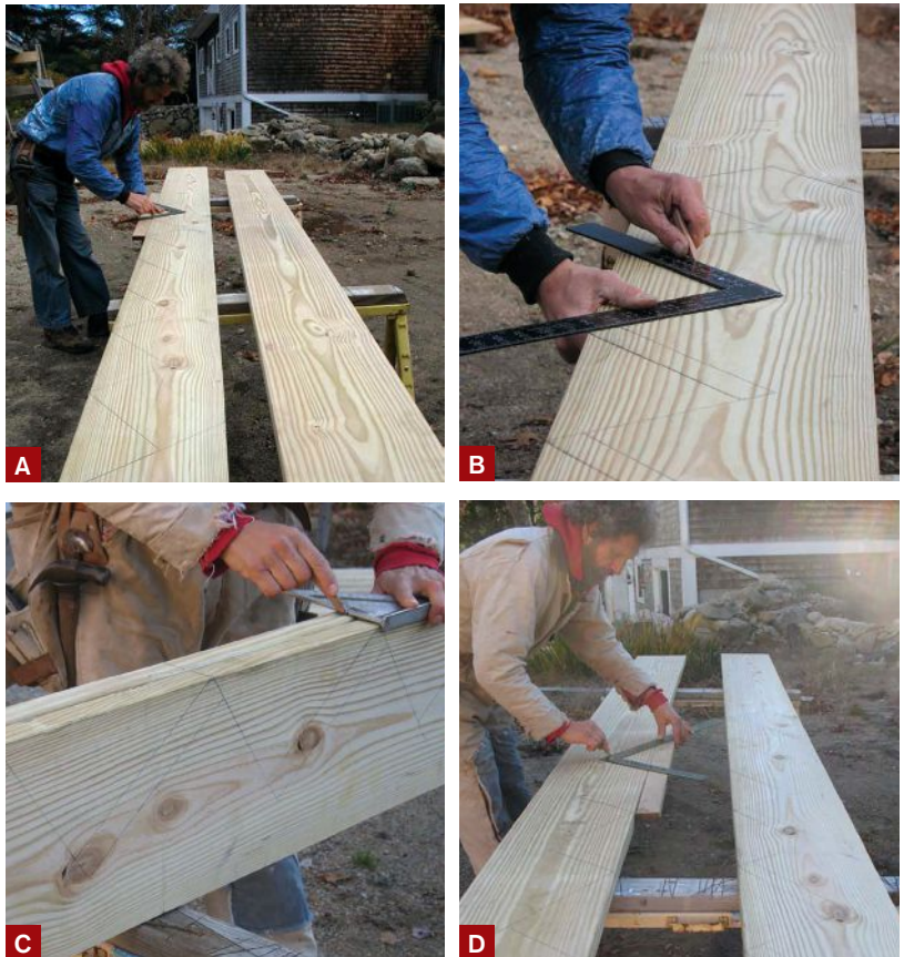
Figure 2. For laying out treads and risers on a pattern stringer, a 1-by straightedge screwed to a framing square provides more accuracy than stair gauges (A). To locate the metal stair brackets, mark both the tops and bottoms of the treads (B). Tilt the two stringers on edge to transfer the tread-riser intersection to the other stringer (C), then lay out the remaining stringer so that it is a mirror image of the pattern (D).
