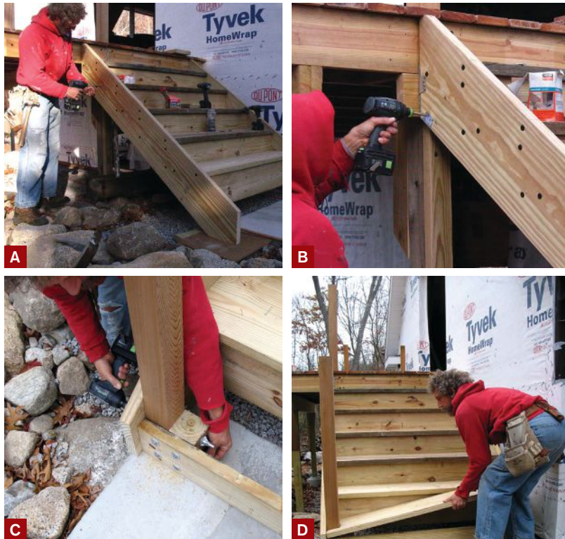
Figure 5. Flat-head structural screws driven through pilot holes in the stringers and into the treads and risers draw the assembly together (A). After the author slides the stairs over into position, he uses stair-stringer connectors to hang the stairs from the rim board and 2-by header (B). ThruLok screws and a hefty blocking detail fasten the guard post to the stringer and the structural riser (C). The final tread is notched to fit around the post, then fastened in place with structural screws (D).
