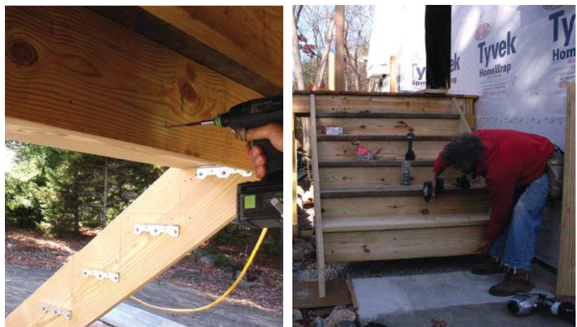
Figure 4. Five-inch-long structural screws driven through the risers into the back edge of the treads 12-inches on-center reinforce the treads (above left). The front edge of the treads and the top edges of the risers are also fastened together with long structural screws (above right).
