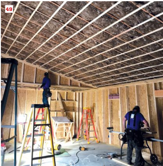
On the cover: Carpenters Alex Strugatskiy and Ryan Bielenda, of Maine Passive House, site-assemble a heavy LVL carrying beam for a custom home in Greenwood, Maine. See the story on page 39. Photo by Ted Cushman.
