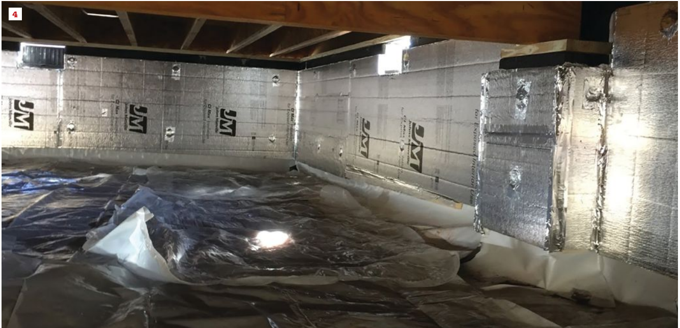
The walls of the crawlspace shown above have been insulated and waterproofed, and a temporary ground cover is in place. Temporary foundation wall vents are left open until the house is drywalled, power is turned on, and the HVAC system is operational so that the space can be conditioned.
