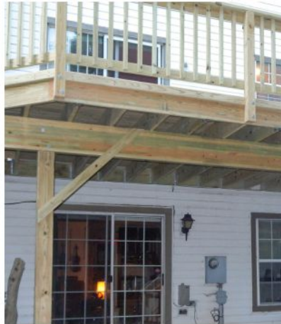
Cantilevered deck joists act like levers, creating uplift where they are attached to the ledger when loads are applied to the cantilevered portion of the deck.
