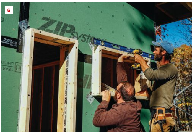
Concrete “cookies” used to brace the wall framing were only partially effective (4). Kelly taped the sheathing joints at openings (5) before screwing on window bucks (6).
