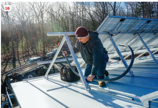
Kelly saved cost by installing the PV brackets and panels (14) and making some of the basic wiring connections himself (15). Electrician Joe Sewell oversaw the work (16).
