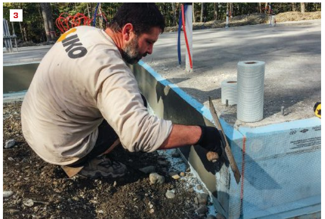
The slab detail was familiar to trade contractors (1), but the radiant-slab tubing (2) was time-consuming. The conventional slab edge detail (3) received an economical stucco finish.
