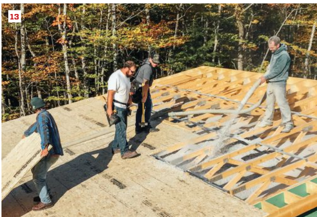
The high-performance roof proved economical. Setting the monopitch trusses (11), installing the OSB air barrier (12), and insulating from above (13) all went quickly.
