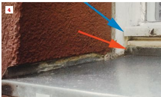
Water details in masonry buildings. Caulk alone (1)? Nope. This end dam (2) is better, but water can leak behind it. On this end dam (3), the stucco covering it will wick water. The last option (4) is the best but is still not perfect. See why?
