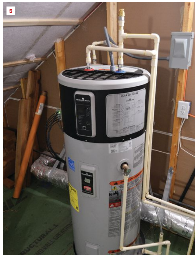
A large jump duct in the attic floor allows free airflow between each bedroom and the buffer space for pressure relief (4). A heat-pump water heater (5) recovers latent heat from the indrawn air, helping to dehumidify the space as it heats water.
