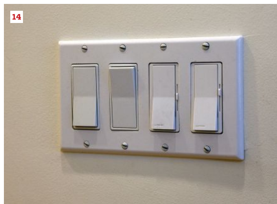
In a bank of switches at the entry to a kitchen, the first switch should always control the ambient lighting (12). Switches near the sink control over-sink lights, while adjacent switches are for under-cabinet lights (13). Keep dimmers together, if possible (14).
