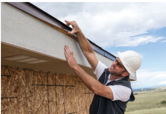
Colorado Springs builder Andy Stauffer installs a screened vent in the soffit of a home near the city (top), then places an outlet vent in the home's roof (middle). At the roof edge (bottom), metal drip edge will extend down into the gutter.
