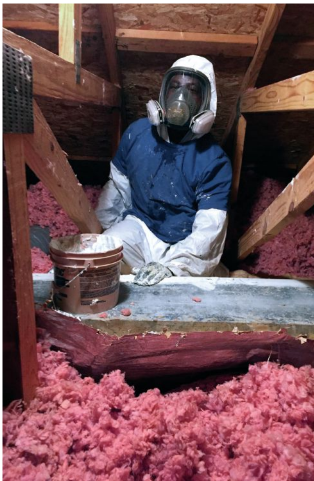
An Edge Energy installer seals a trunk line in an existing home before burying the duct with blown cellulose—a safe and routine practice in mixed climates, says Gary Boyer.
