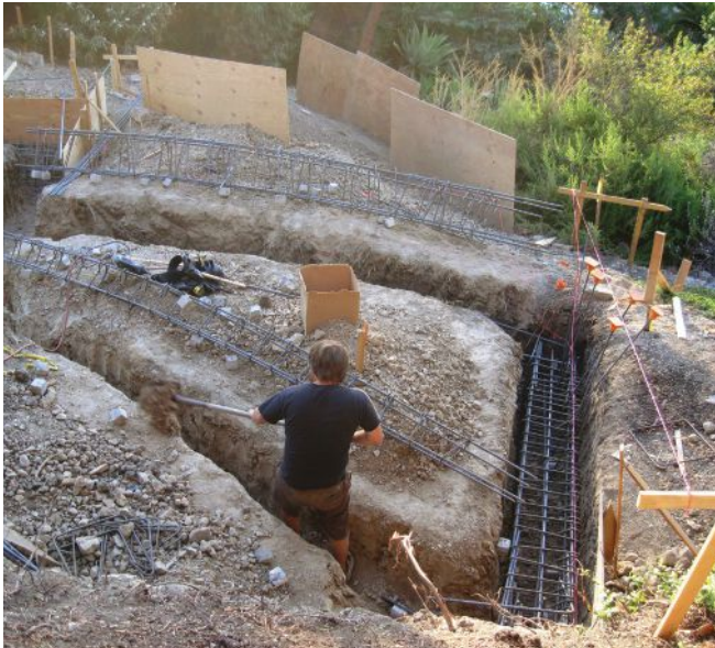
Above, a worker shovels out the trench for grade beams that will support the stem wall for the unconditioned crawlspace under Sylvia Wallis' addition.
