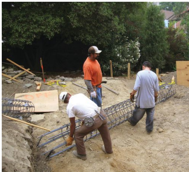
Above, foundation workers set rebar cages for deep structural piers into the hillside for Sylvia Wallis’ high-performance addition.
