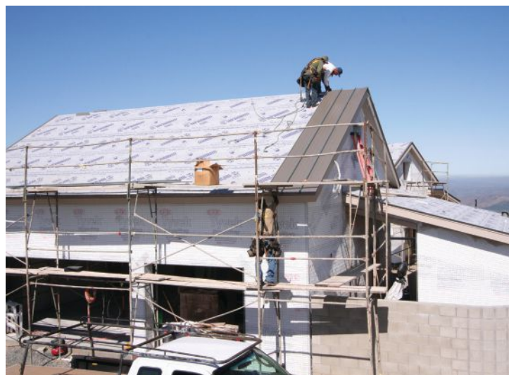
Carpenters apply 6-inch SIPs to the roof frame (top). The roof sheathing under the SIPs has already been air-sealed with fluid-applied membrane. Above, roofers install steel roofing panels on top of synthetic roofing underlayment.
