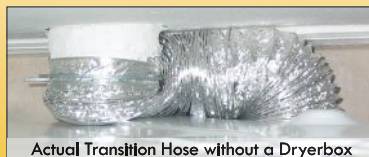
Actual Transition Hose without a Dryerbox
