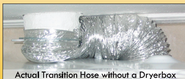
Actual Transition Hose without a Dryerbox
