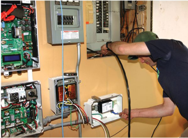
Scott Millette pulls cable into the smart meter box from the home's main panel. To the left of the panel is the load center with breakers serving the home's backed-up circuits.
