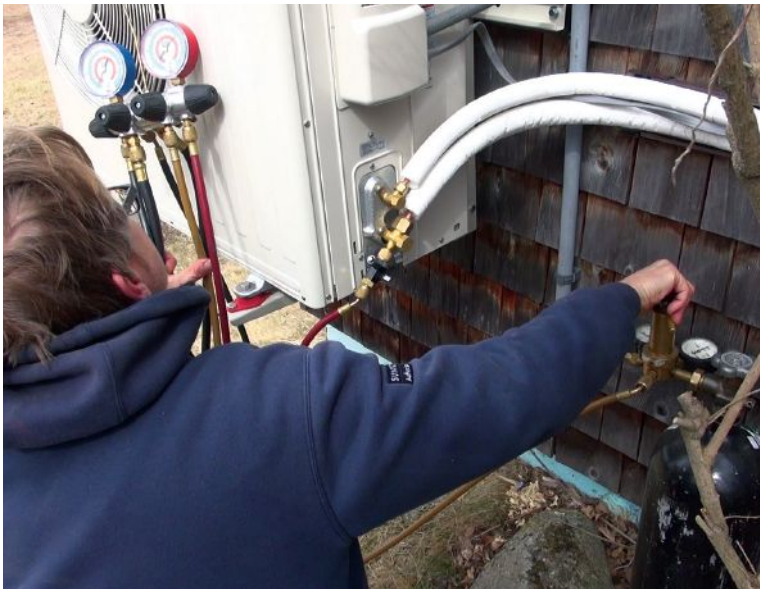
ReVision Energy tech Dave Ragsdale sets up equipment for the pressure test and triple-evacuation refrigerant-line-clearing procedure for a newly installed Mitsubishi mini-split at a rural home in Maine.
