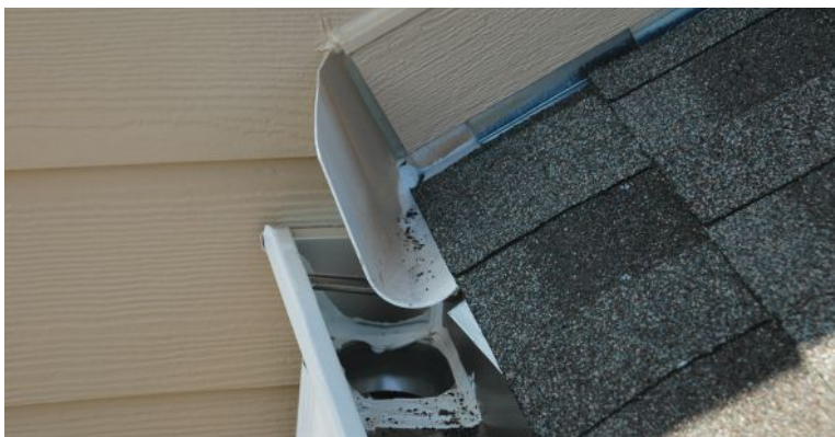
With horizontal siding, the author installs a trim board along the rake, keeping it a minimum of 1 inch above the roofing.
