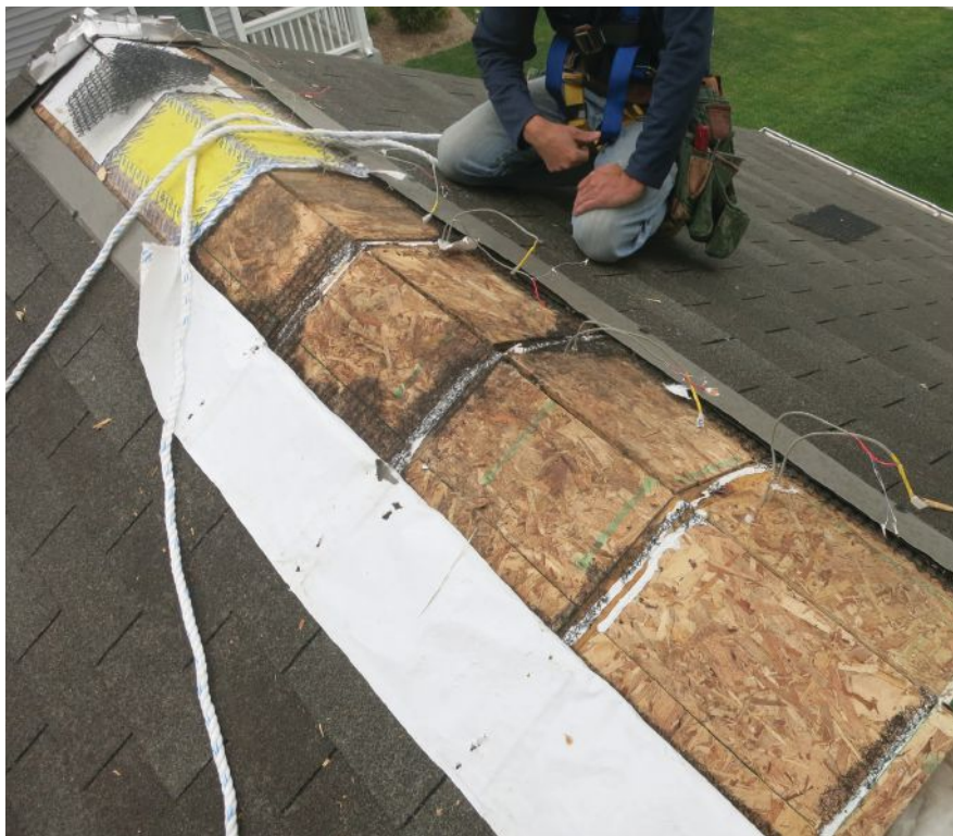
Insulated cathedral roof bays are exposed as part of a side-by-side test of various insulation and venting options under real-world conditions. Ventilation has obvious benefits, Kohta Ueno reports, but some unvented solutions can work.
