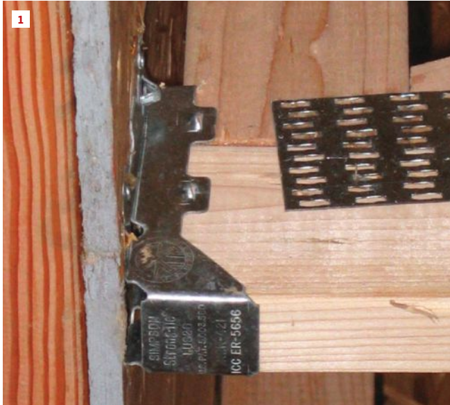
The gap at the end of the floor truss is a tell-tale sign of a framing violation. Any truss or joist must have full bearing on the hanger seat. This hanger may be undersized, as well, for the size floor truss it supports.
