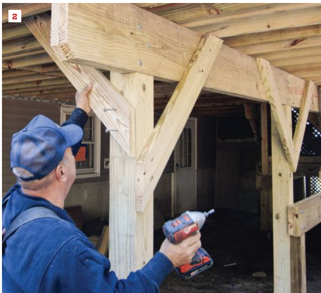
Racking resistance is a structural key to a deck that will resist failure over time. This photo shows an effective way to brace deck posts. Running the diagonals in both directions provides much-needed racking resistance.
