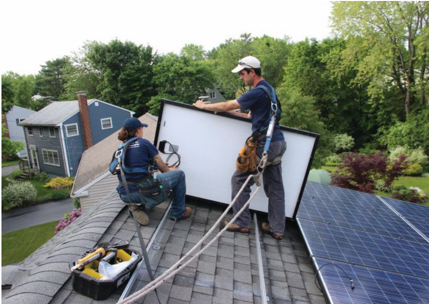
Technicians for Revision Energy install PV panels for a grid-tied system on a Portland, Maine, roof in 2014. A panel array this size might supply all the power a house needs on a net annual basis, but still requires a grid connection to balance surplus summer production against nighttime and winter power needs.
