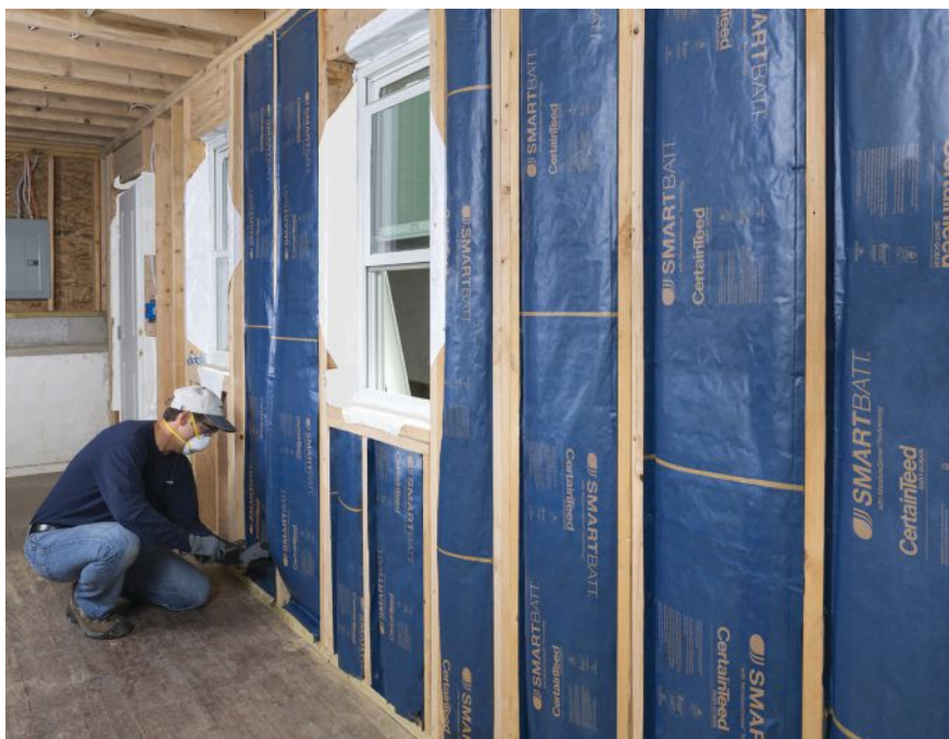
A worker installs CertainTeed SmartBatt fiberglass batts into a stud cavity in this photo supplied by CertainTeed. Applied in this manner, the product helps manage vapor diffusion, but will not serve as an air control layer.
