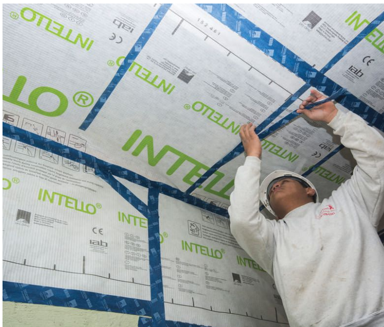
A technician for J’s Custom Contracting installs Intello smart vapor barrier on the ceiling under the low-slope roof of a Brooklyn, N.Y., row house. Flat roofs, which are tricky to vent, are one case where smart membranes can be problem solvers.
