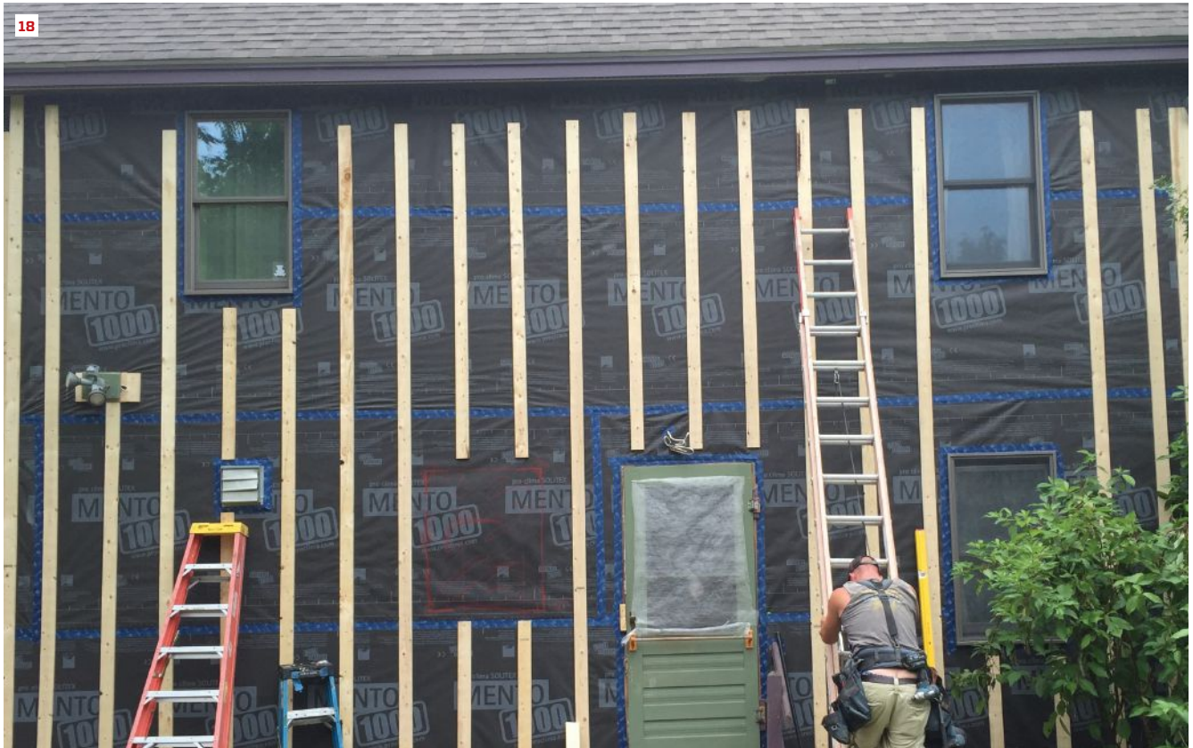
Over the vapor-open Solitex Mento 1000 weather-resistant barrier, the crew applied 1x4 strapping to create an air channel behind the new fiber-cement lap siding (18).
