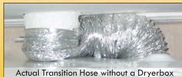
Actual Transition Hose without a Dryerbox
