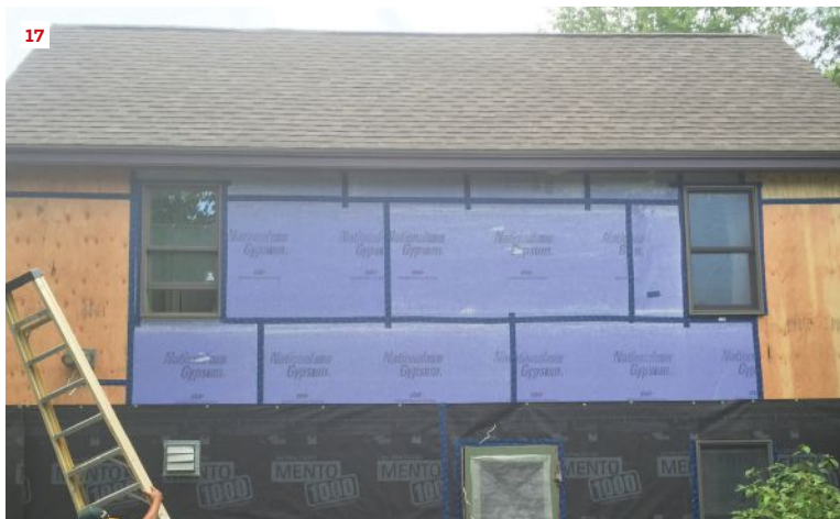
After resheathing the newly insulated walls with vapor-open Gold Bond gypsum board (15) and taping the seams with Tescon Vana tape (16), the crew covered the sheathing with Solitex Mento 1000 (17).
