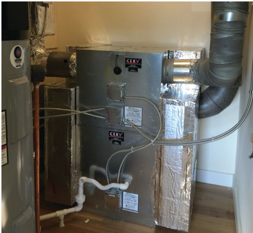
A Build Equinox Conditioning Energy Recovery Ventilator (CERV) is shown installed in the mechanicals room of a superinsulated 1,000-square-foot modular home in Vermont. The unit preconditions incoming air and delivers cooled or warmed fresh air to remote rooms as needed, controlling humidity and air quality as well as temperature.
