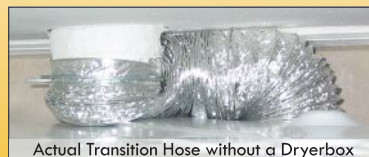
Actual Transition Hose without a Dryerbox
