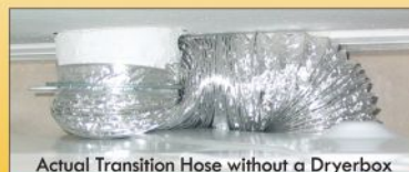
Actual Transition Hose without a Dryerbox
