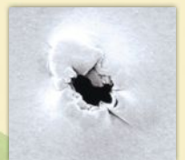
Perforated house wraps enlarged. Holes are large enough to allow water droplets to enter walls.
