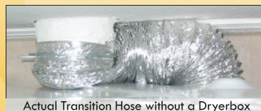
Actual Transition Hose without a Dryerbox
